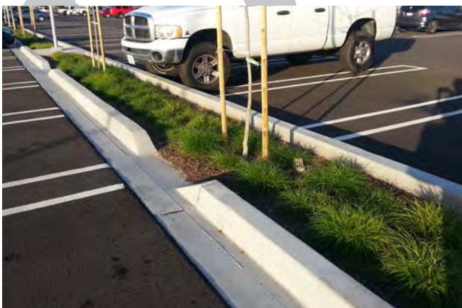
A bioswale in a parking lot can help to reduce stormwater runoff.
