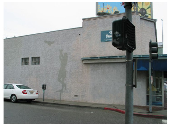
Building needs new paint as well as new “shadow”
