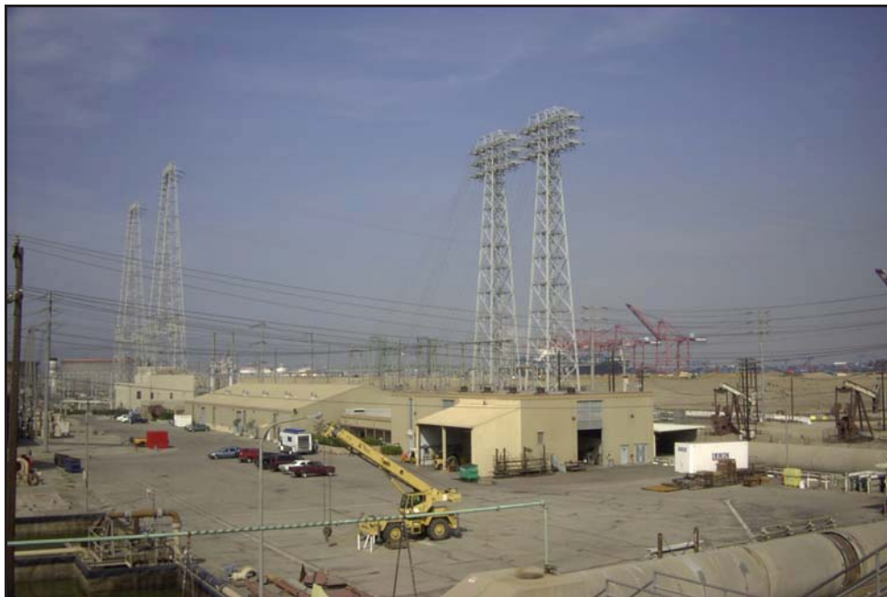
Exhibit 2.1.8-2 Photograph of Transmission Towers
