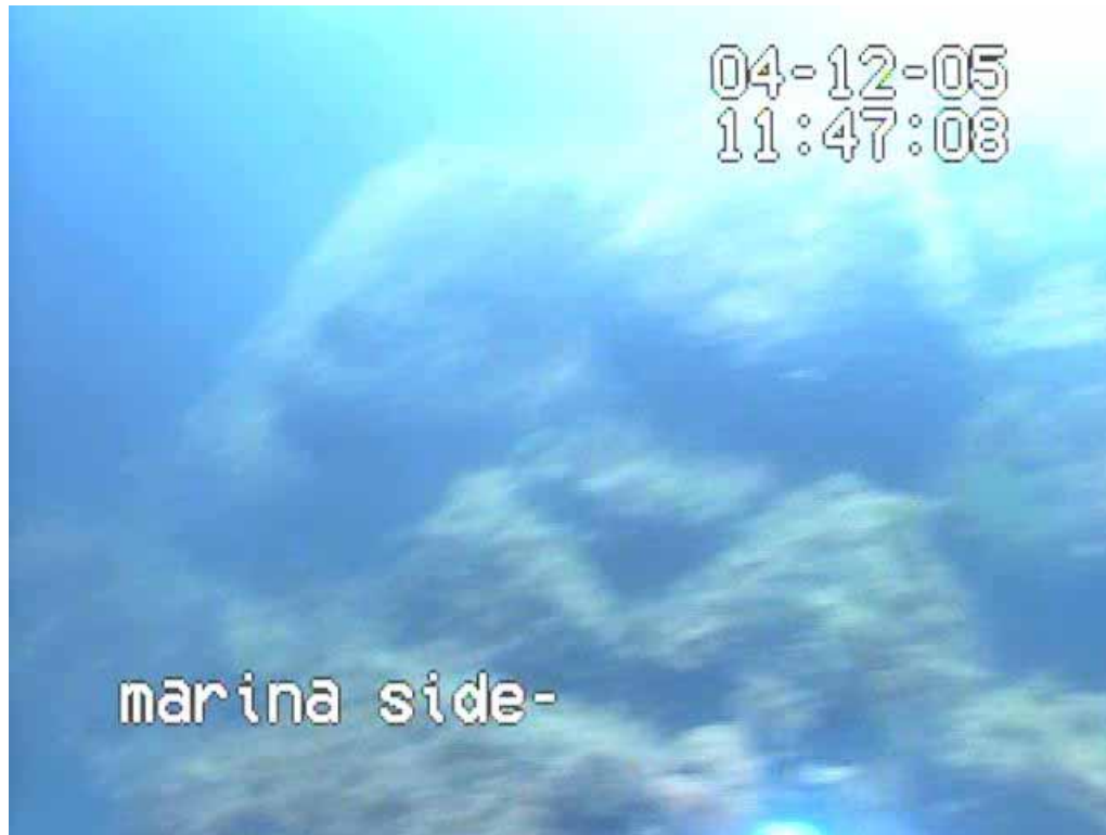
PHOTO 5 - ROCK BUILD UP OUTSIDE OF MARINA OPENING. THIS PILE IS IMPEDING FLOW AND IS 3.5' HIGHER THAN THE CULVERT FLOOR AND IS ABOUT 6' WIDE
