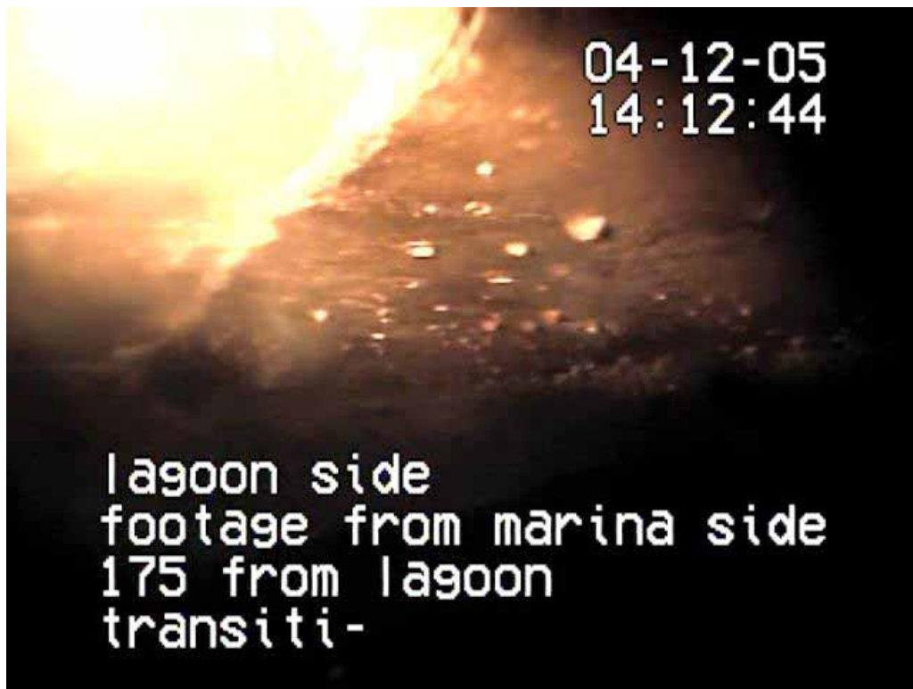
PHOTO 8 - SHOWING START OF TRANSITION. THE EDGED CONCRETE IN ON THE LEFT CENTER IS THE START OF THE TRANSITION WHERE THE TOP OF THE CULVERT LOWERS
