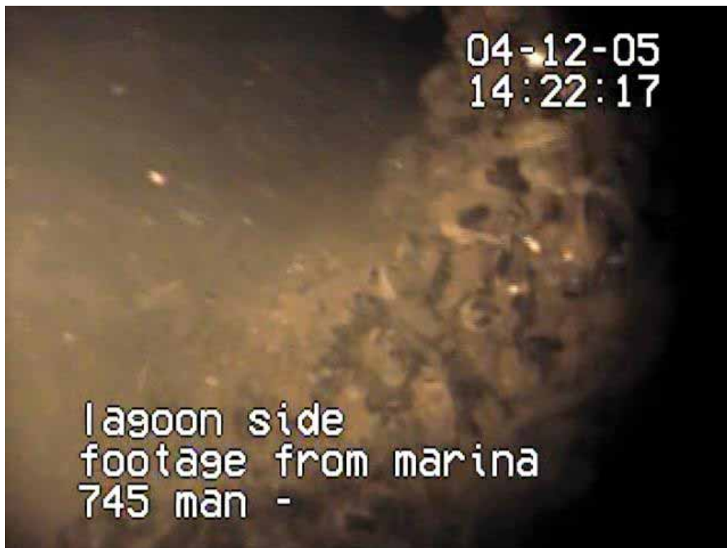
PHOTO 10 - 30" DIAMETER PIPE IN NORTH WALL APPROXIMATELY 755 FEET FROM THE MARINA SIDE. THIS IS THE FIRST OF TWO PIPES
