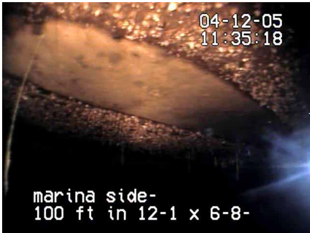
PHOTO 6 - TYPICAL OVERHEAD SHOT SHOWING BIOFOULING AND TYPICAL CONDITION
