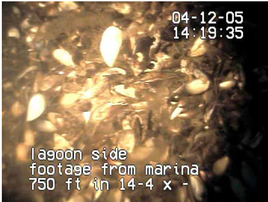
PHOTO 9 - TYPICAL MATERIAL BUILD UP SHOWING THE SHELL MATERIAL FOUND ON THE FLOOR
