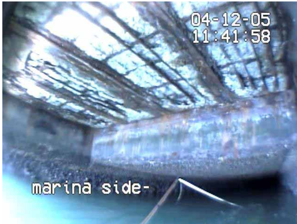
PHOTO 3 - EXPOSED REBAR AND MISSING CONCRETE AT MARINA SIDE COVERS, LOOKING FORWARDS THE LAGOON
