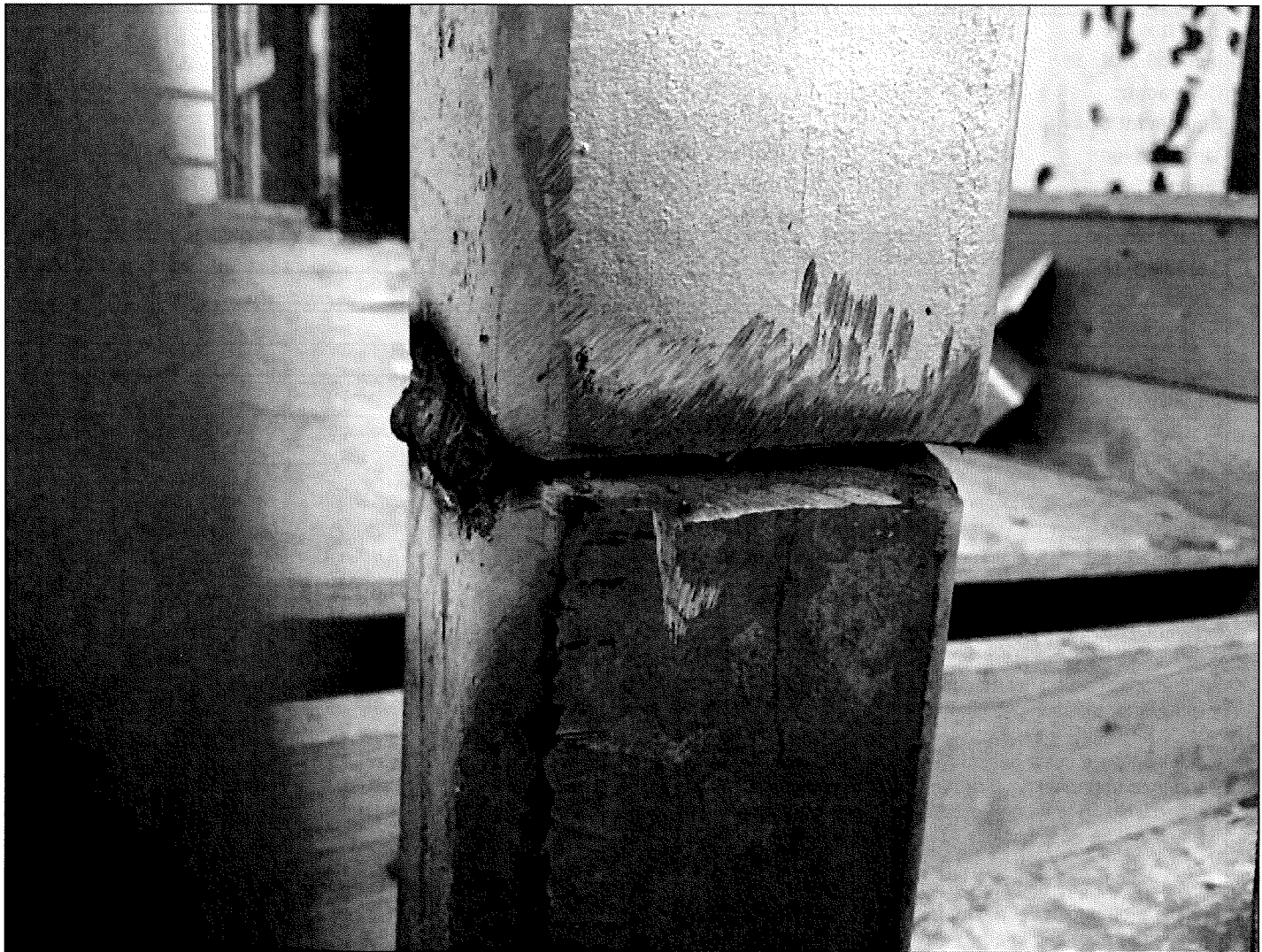
Incompleted welds that could be done with out crane
