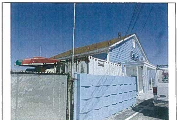
Figure 9: North elevation, looking south, view obscured by fence and storage. Source: GPA.
