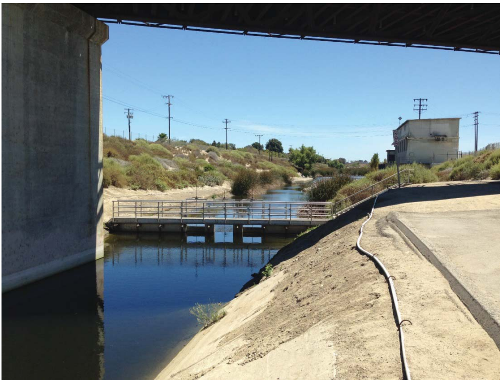
Photo 4: Looking south towards weir and pumping station in the Dominguez Gap Wetlands, with UP railroad track bridge overhead in foreground.
