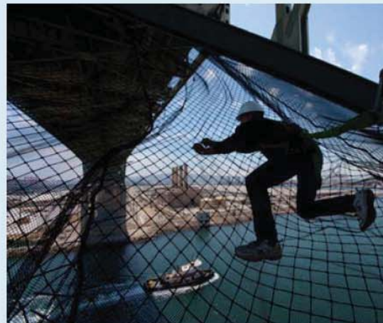
A worker repairs netting (known as a “diaper”) below the bridge that stops broken pieces of concrete from falling.
