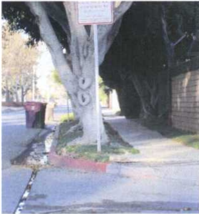
Tree root damage to sidewalk
