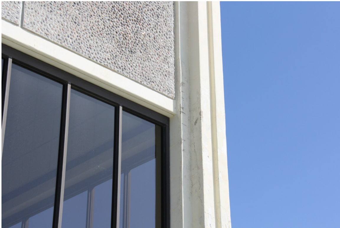
Figure 22 – Natatorium Building, Cracks in Column at Southeast Corner (Grid H/18)
