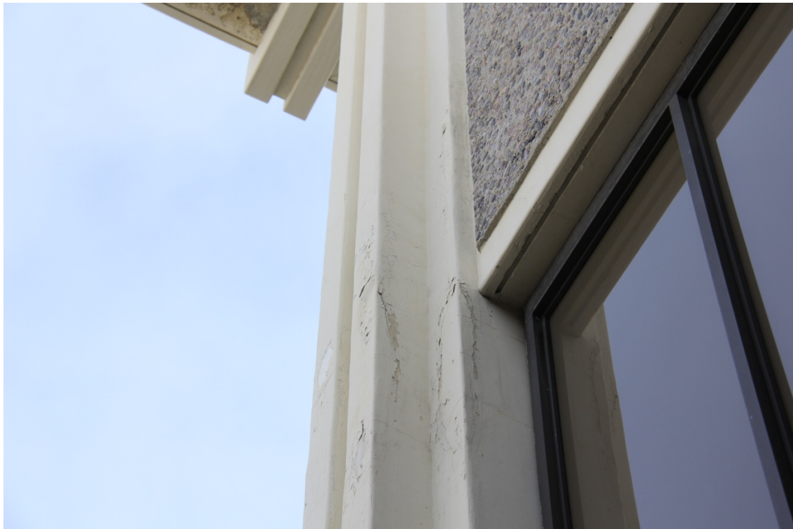
Figure 16 – Natatorium Building, Cracks in Column at Northeast Corner (Grid A/7)
