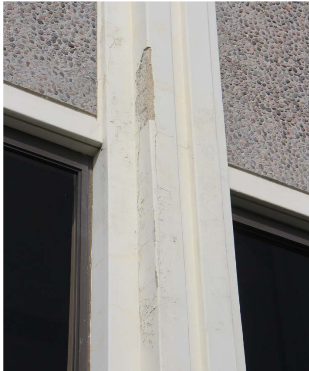
Figure 19 – Natatorium Building, Cracks in Column at East Elevation (Grid B/18)
