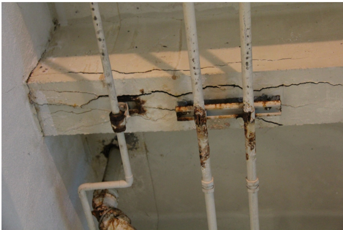
Figure 28 – Community Building, Cracks in Concrete Beams in Basement
