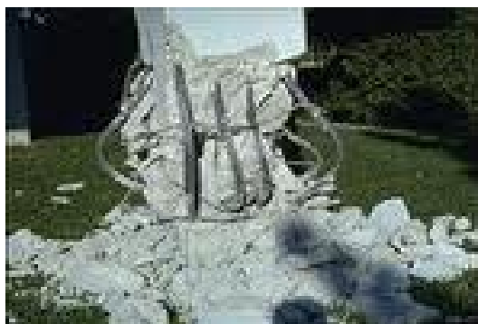
Photo 4 – Imperial County Service Building, 1979 Earthquake Damage
