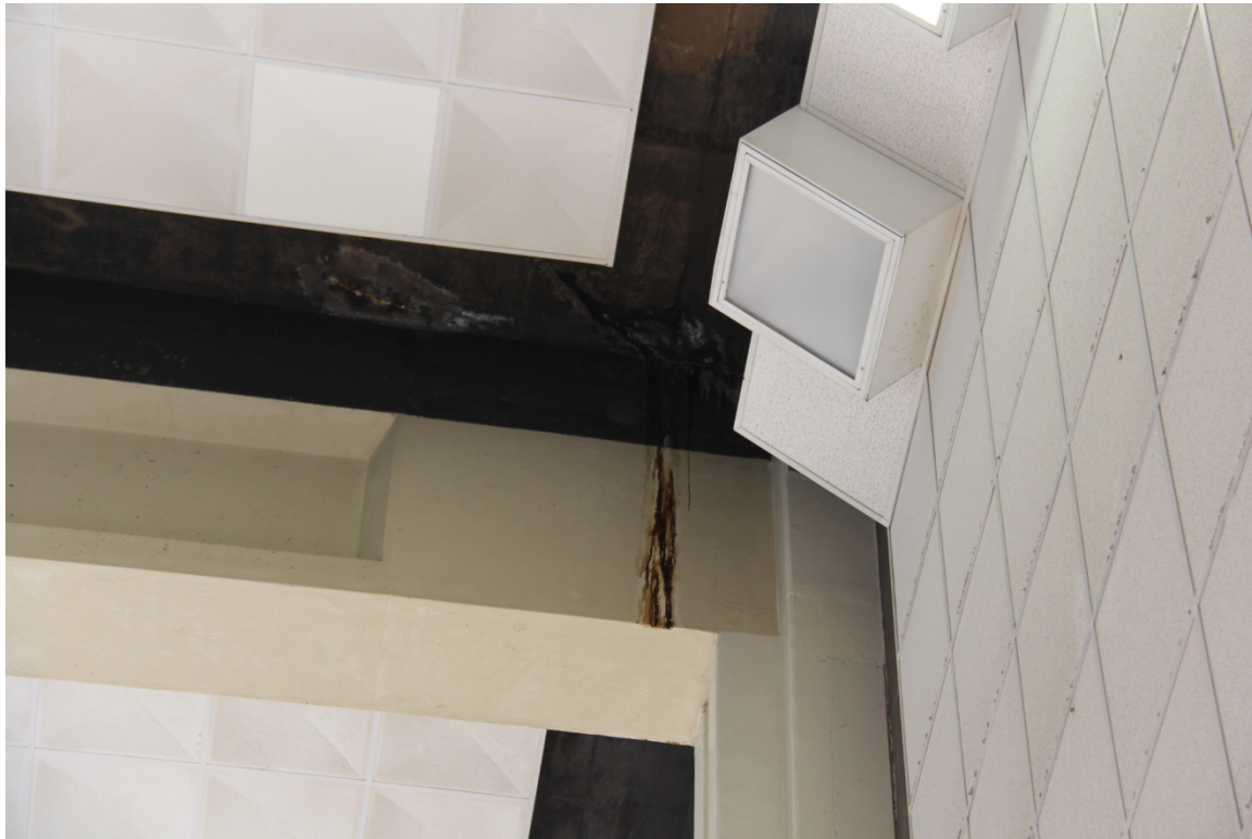
Figure 25 – Natatorium Building, Stains in Roof Slab/Beam at Interior South End
