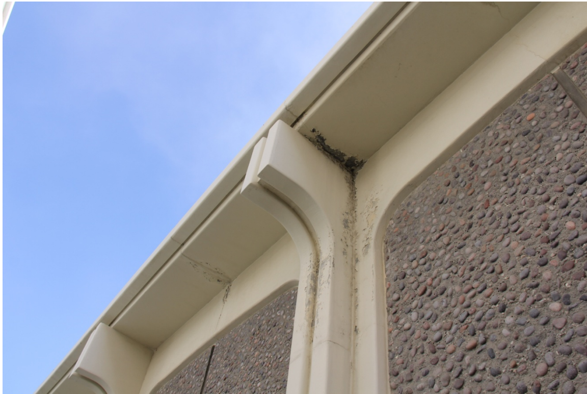
Figure 27 – Locker Building, Cracks in Concrete Roof Slab at West Elevation
