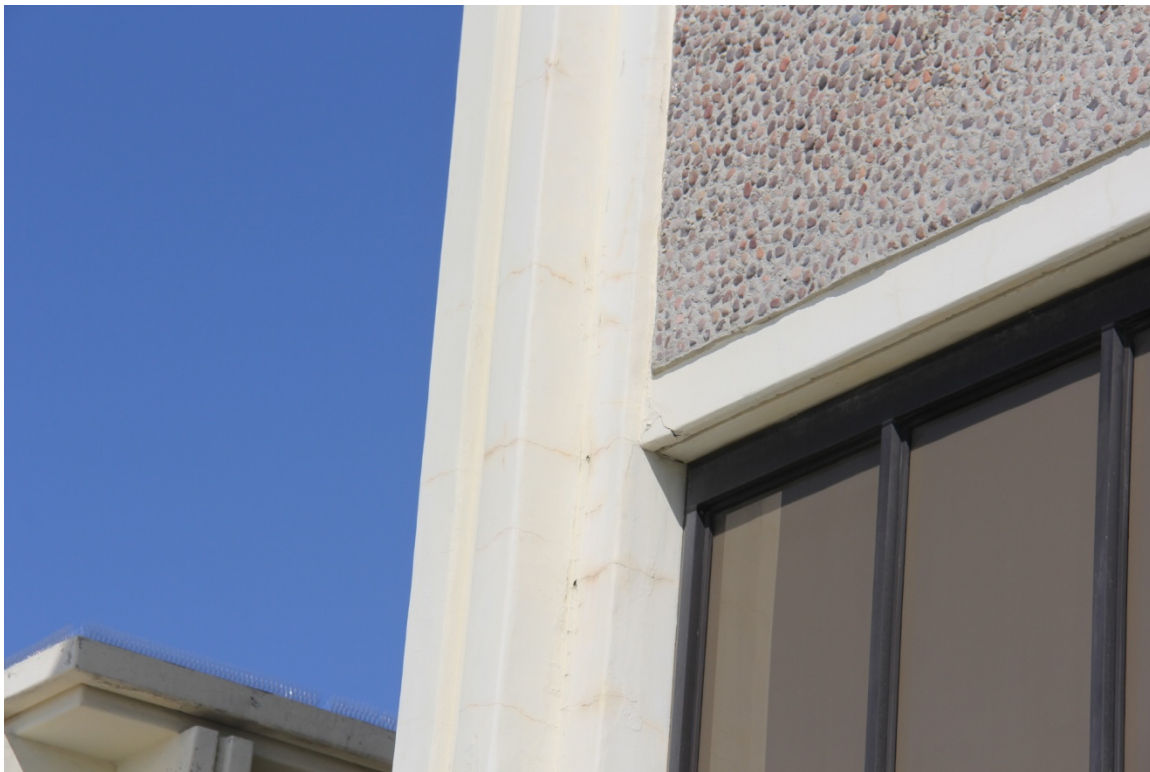
Figure 24 – Natatorium Building, Cracks in Column at Southwest Corner (Grid H/7)
