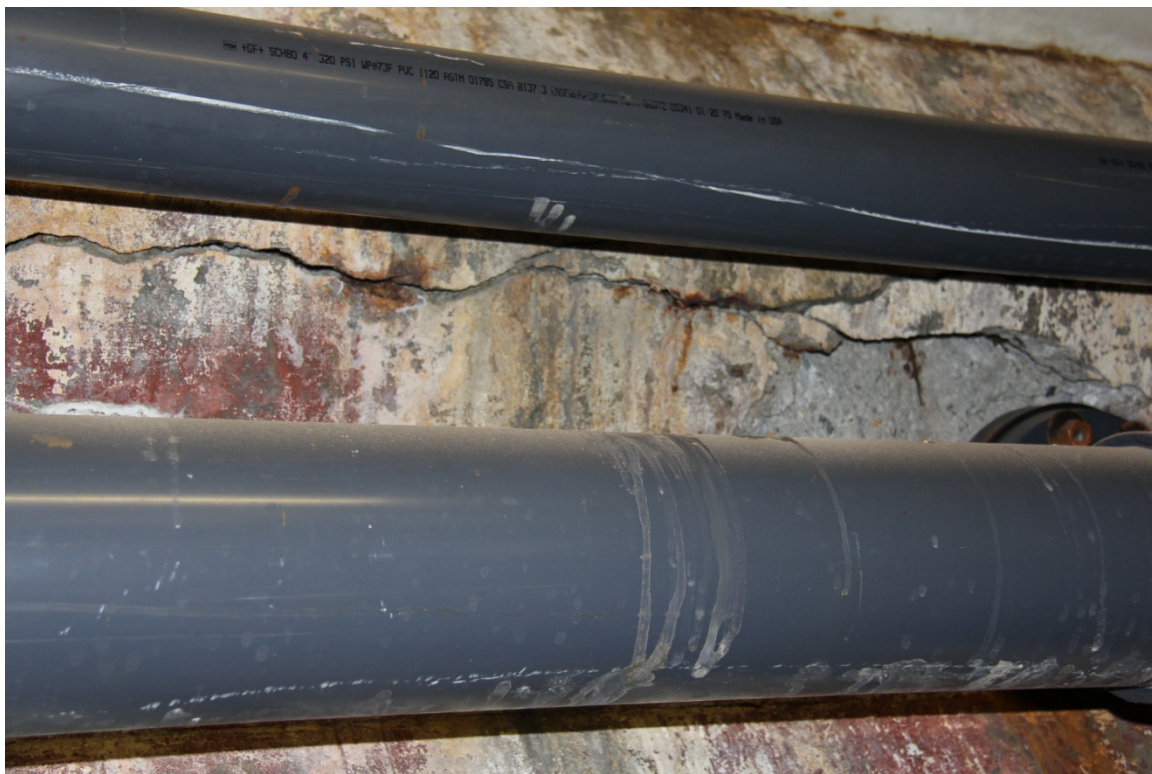
Figure 30 – Community Building, Cracks in Concrete Wall in Basement
