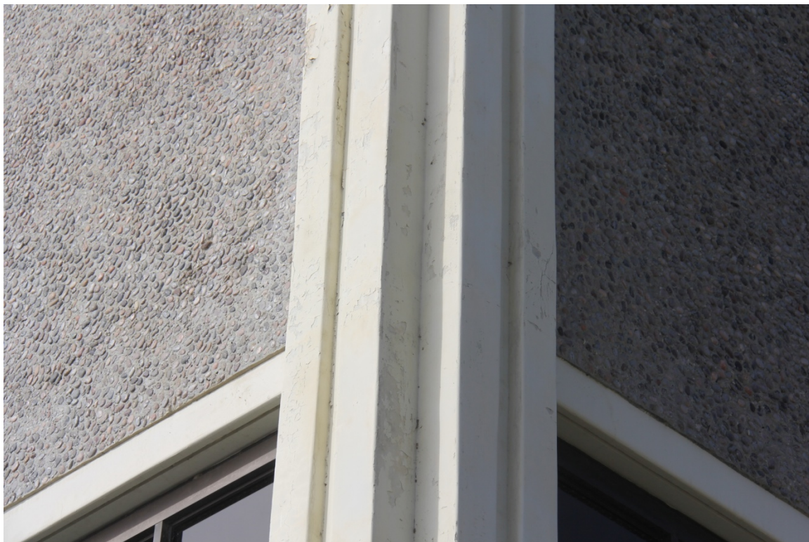
Figure 18 – Natatorium Building, Cracks in Column at Northeast Corner (Grid A/18)
