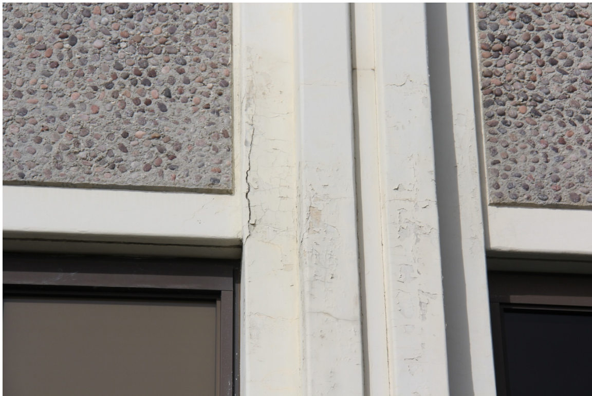
Figure 20 – Natatorium Building, Cracks in Column at East Elevation (Grid C/18)
