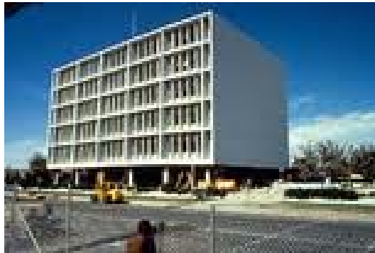
Photo 1 – Imperial County Service Building, 1979 Earthquake Damage
