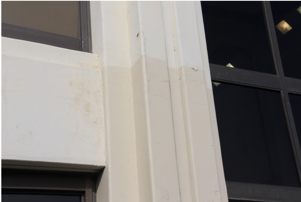
Figure 21 – Natatorium Building, Cracks in Column at East Elevation (Grid C/18)
