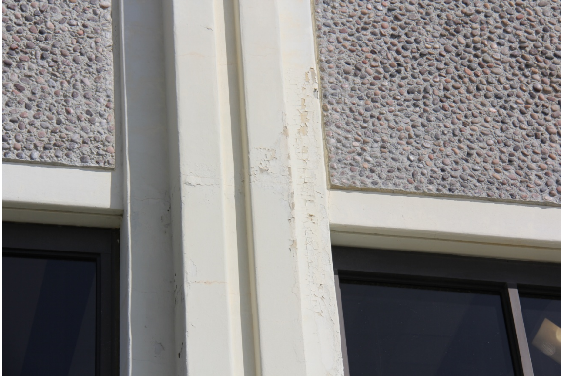
Figure 23 – Natatorium Building, Cracks in Column at South Elevation (Grid H/17)
