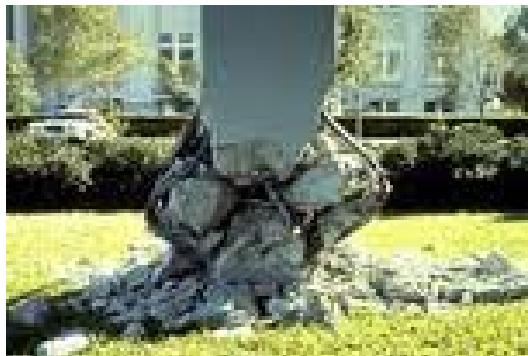
Photo 3 – Imperial County Service Building, 1979 Earthquake Damage
