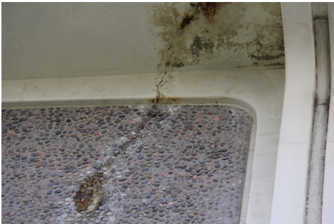
Figure 26 – Natatorium Building, Cracks in Concrete Wall/Roof at North Elevation
