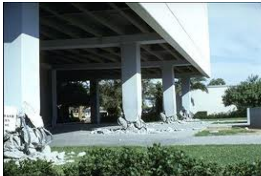
Photo 2 – Imperial County Service Building, 1979 Earthquake Damage
