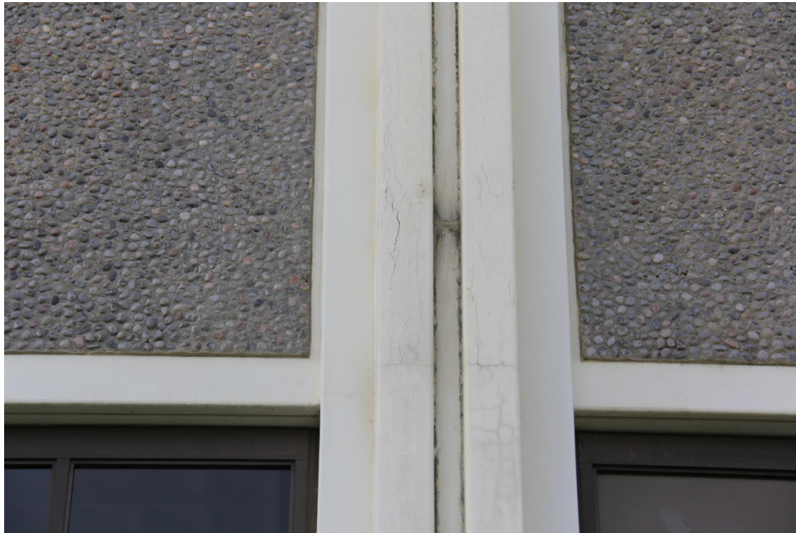
Figure 17 – Natatorium Building, Cracks in Column at North Elevation (Grid A/11)
