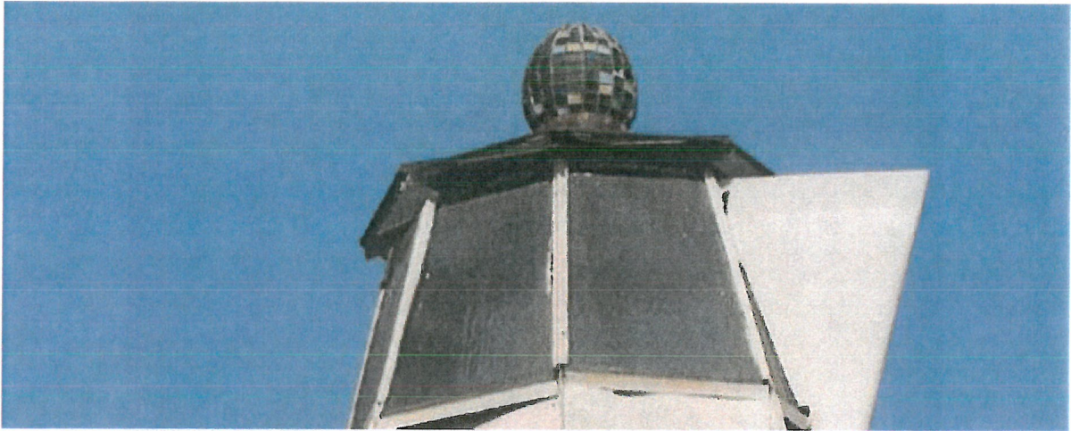
View of Missing Knob, Photograph: RoadArchitecture.com, dated March 24, 2008
