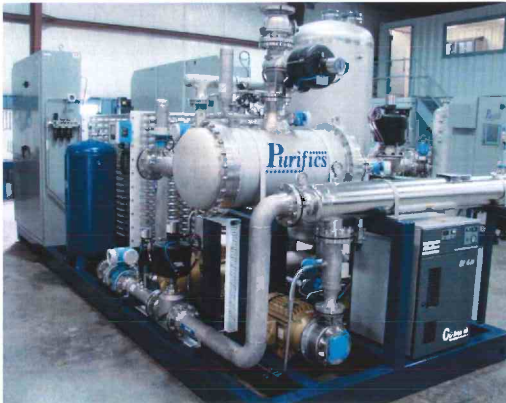
Figure 2: Photo-Cat AOP+ Drinking Water System for 1,4-Dioxane and cVOC Destruction
