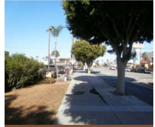
Figure 2.30 Indian Laurel Fig (ficus) trees along Broadway, showing damage to the sidewalk from extensive root systems. Ficus trees should be phased out over time.
