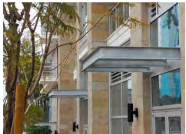
Example of a setback elevation that uses some variation in heights, balconies and materials; the windows and doors are well detailed and noticeably inset. Example of higher quality materials and entrance canopies being used at the ground floor.
