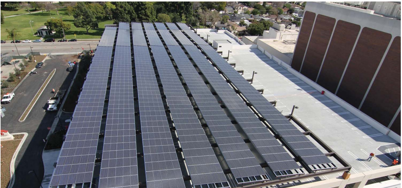
Solar photovoltaic system atop a parking structure at Long Beach City College Liberal Arts Campus.
