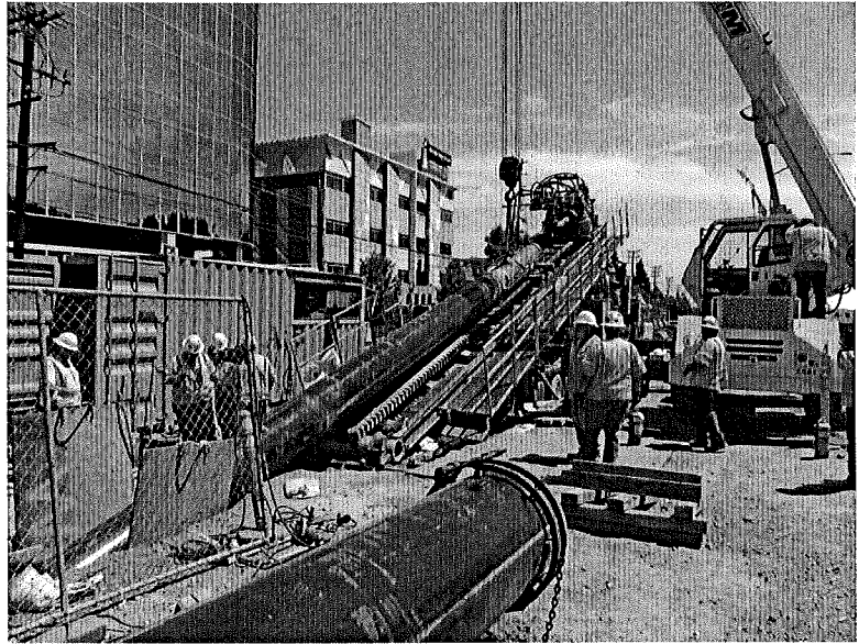
HMM provided third-party coordination for the I-405 Sepulveda Pass Widening Project, including the Chevron Pipeline Relocation shown above.
