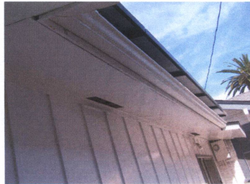
Forcing the array to the back overhangs the gutter, produces less power, and requires trimming of protective trees. The garage floods.
