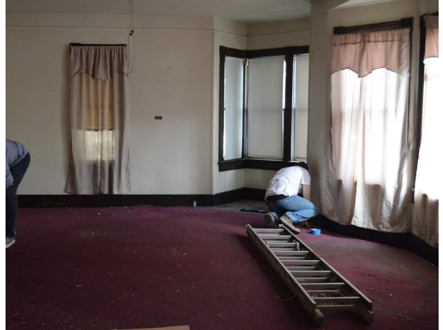
Living room area in Parsonage, First Floor, View West (existing condition) Photo: June 2018
