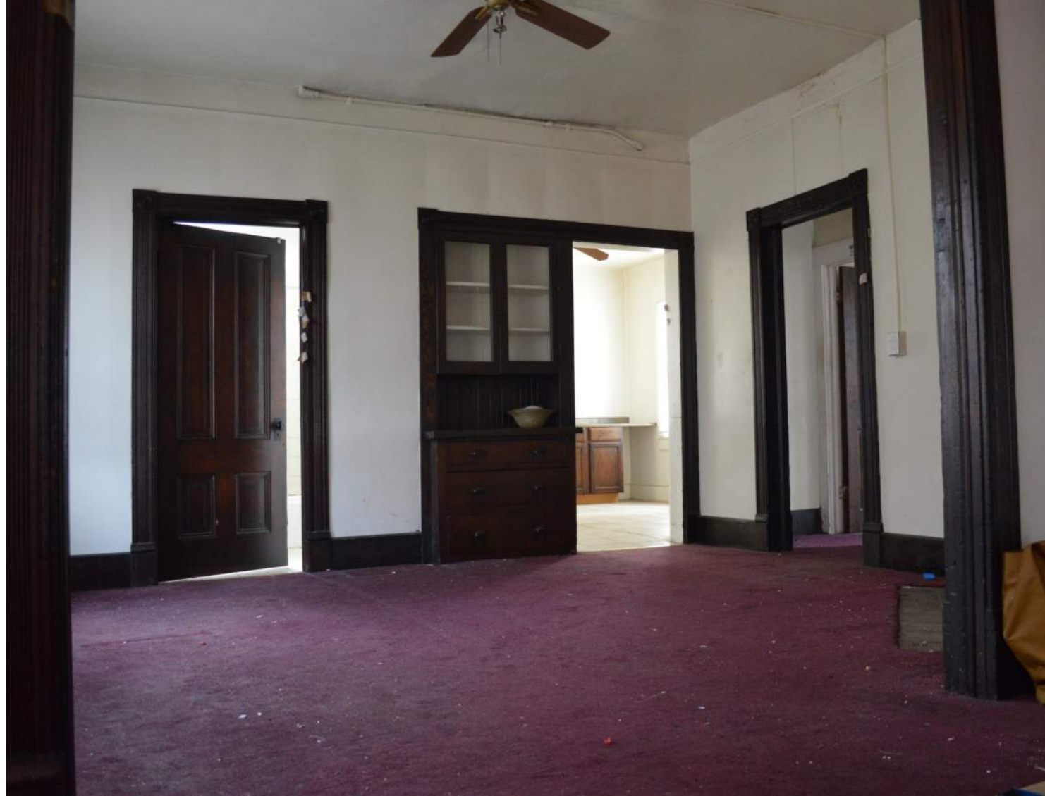
Cabinet and wood detailing in Parsonage dining room, First Floor, View Southeast (existing condition) Photo: June 2018
