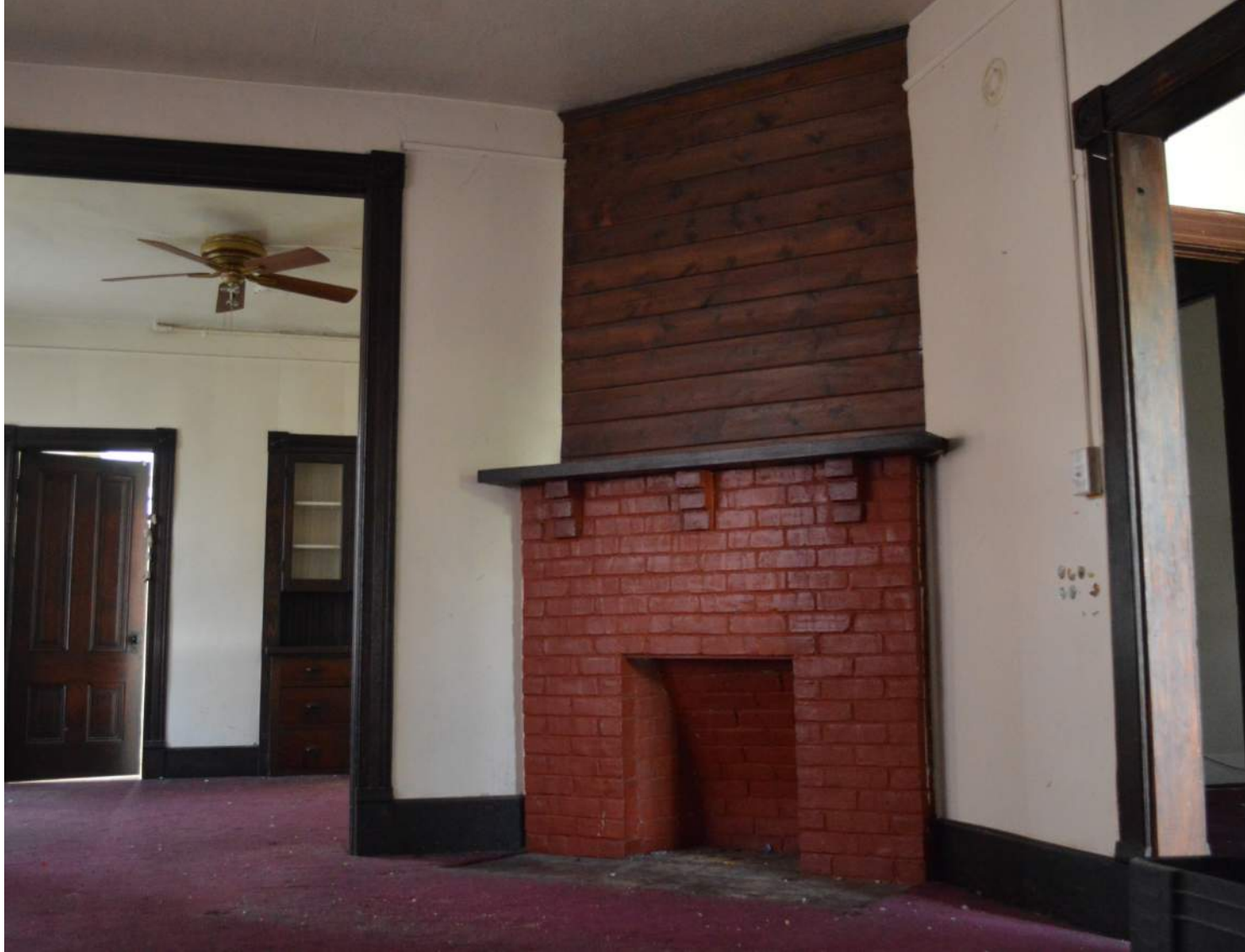
Fireplace and wood trim in Parsonage living room, First Floor, View Southeast (existing condition) Photo: June 2018
