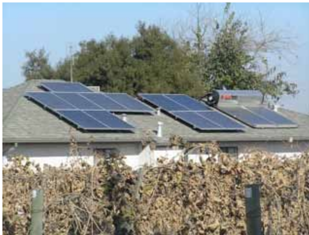
Solar water heating can be found in conjunction with solar electric panels.
