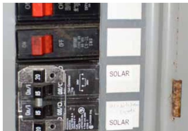
The Utility Group should watch for visual indicators like these warning labels to identify the existence of additional electrical power sources to the building.
