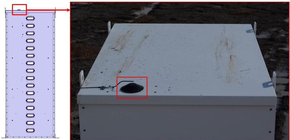
Figure 10 Illustration of the Powerpack exhaust vent (left) and an image of the vent at the top of the Powerpack (right)
