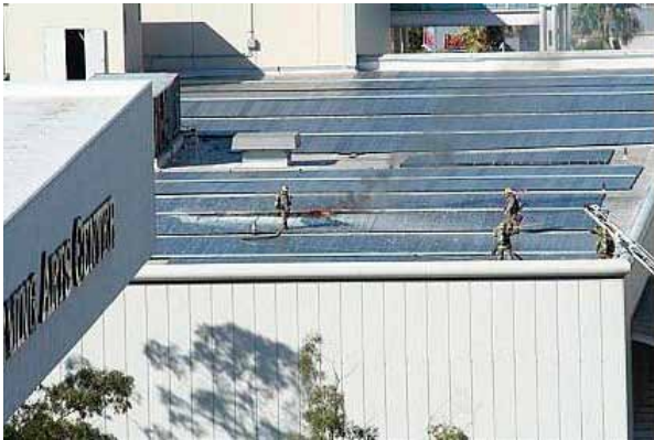
The modules on fire at the Long Beach Convention Center were damaged in shipping and field repaired by the manufacturer's rep prior to installation.
