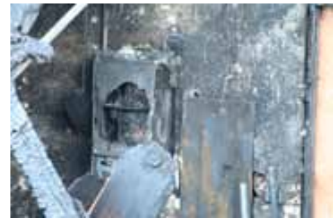
A content fire in the garage of this residence destroyed the PV inverter box.
