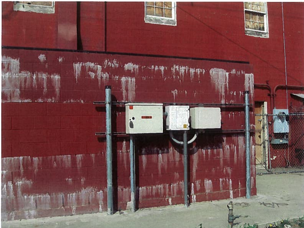
Subject Property – Appurtenant Communication Equipment (T1 Lines)
