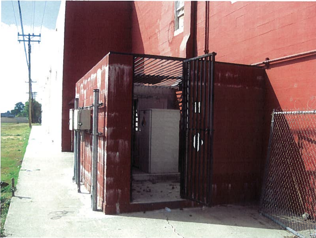
Subject Property – Appurtenant Communication Equipment (Enclosure)
