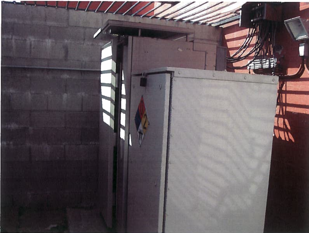
Subject Property – Appurtenant Communication Equipment (Main Cabinet & Backup Battery Cabinet)
