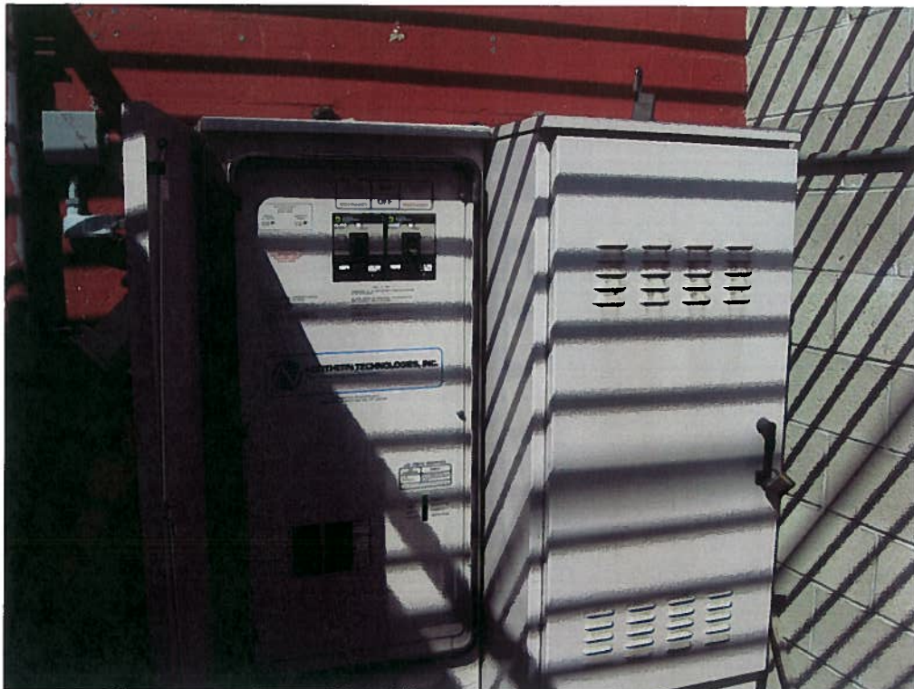
Subject Property – Appurtenant Communication Equipment (Telco & Electrical Cabinet)
