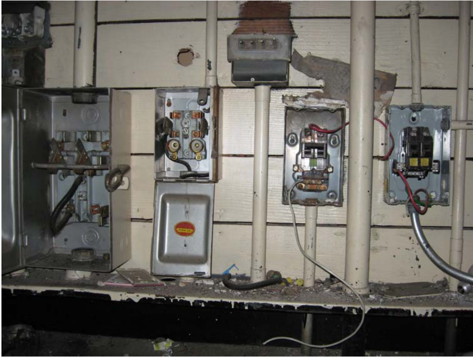
21. Vandalized electrical equipment.
