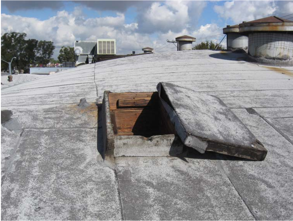
27. Roof hatch is unsafe and not up to code.
