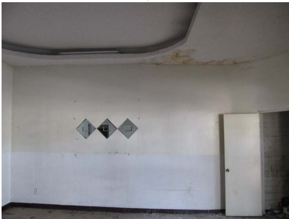
15. Theater interior lobby note water damage at ceiling.
