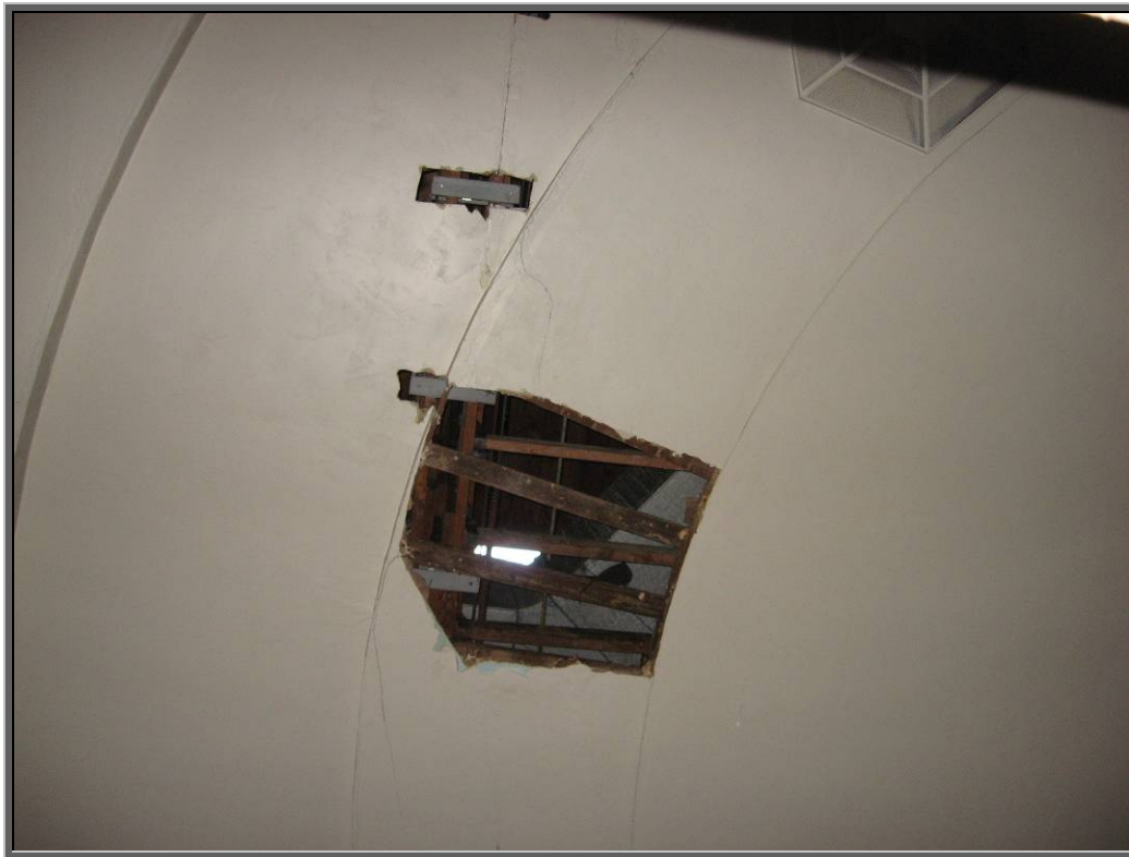
Photo 8: Water damaged plaster ceiling over theater floor.
