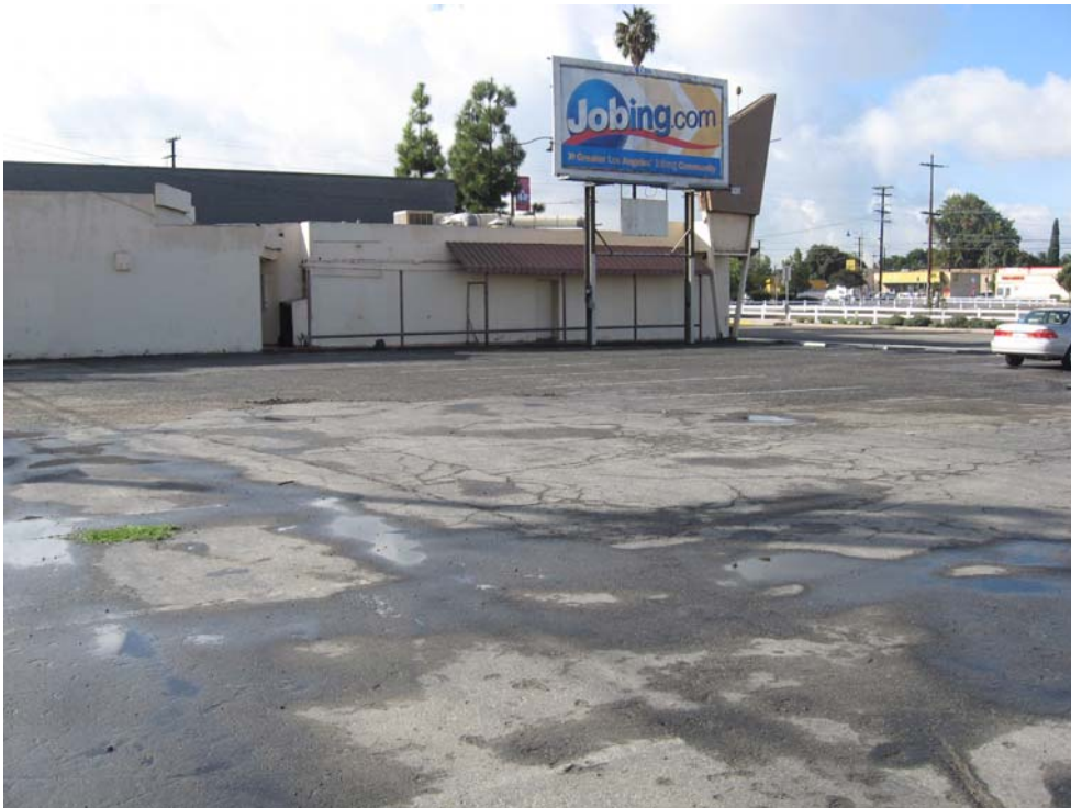
10. Poor condition of asphalt paving.
