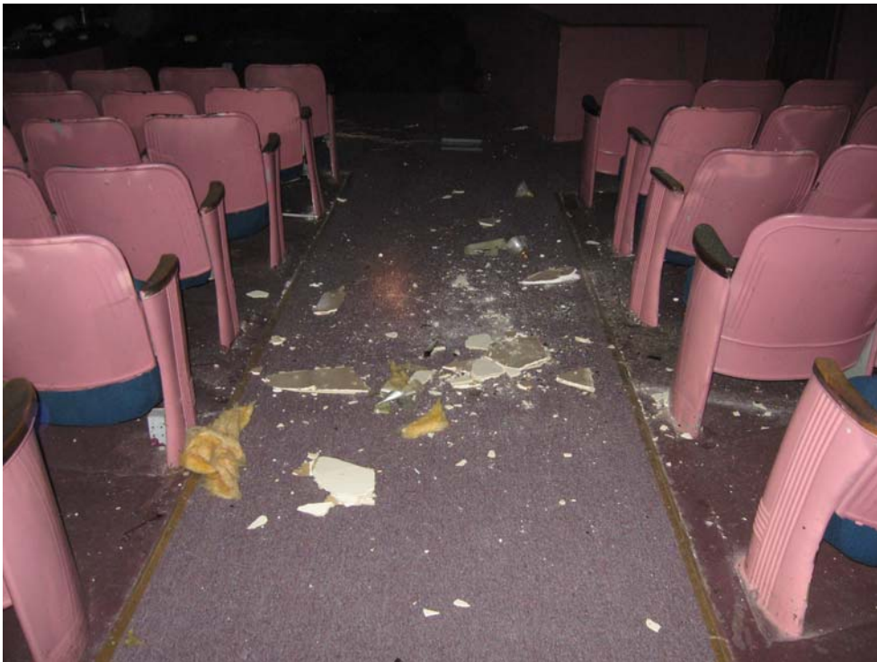
24. Water damage from the ceiling of the auditorium is evident throughout.
