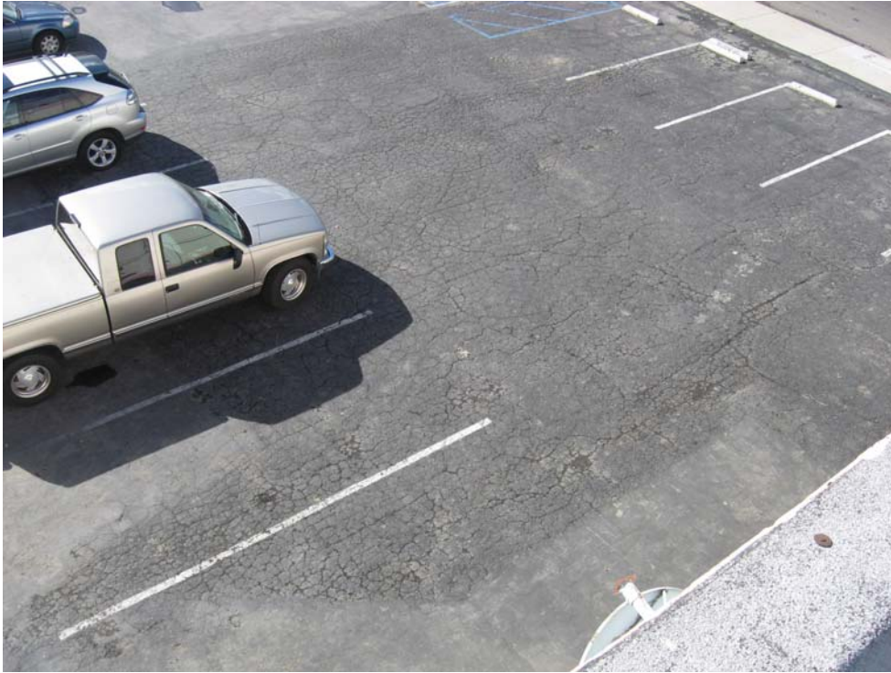
9. Cracks visible throughout the paving.
