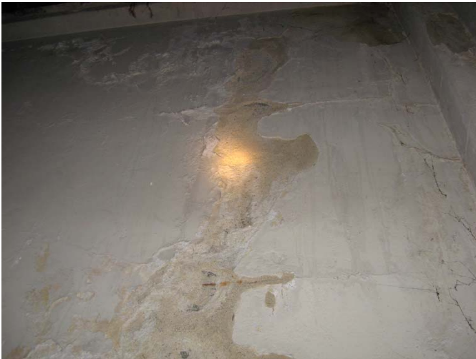
18. Water damage in the interior walls of the furniture store.
