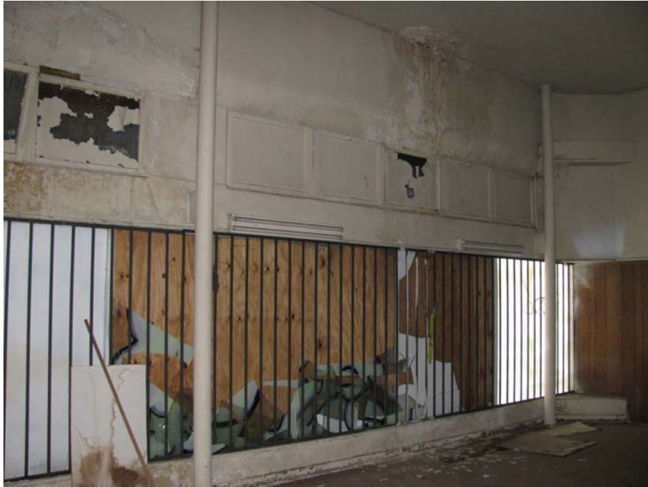
11. Water damage along the interior of the Hanson Building.
