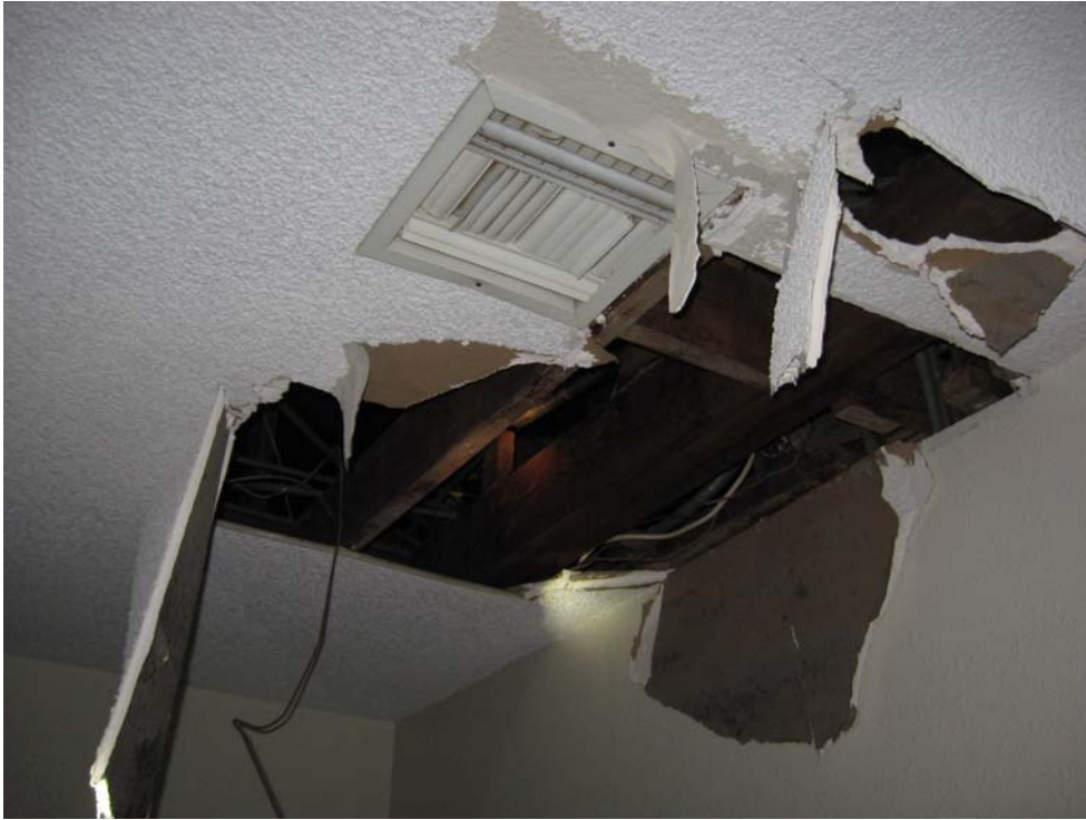
23. Water damage to the ceilings is evident throughout.
