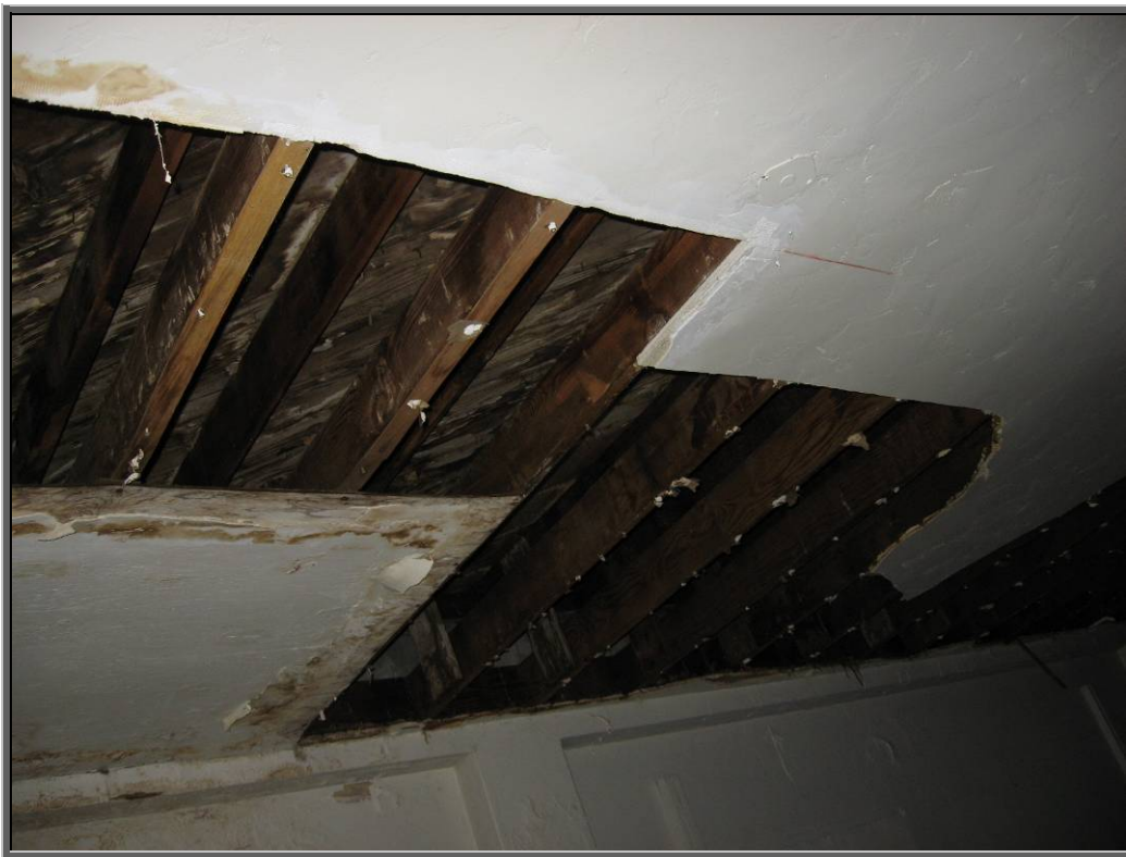
Photo 9: Water damaged plaster ceiling over Hansen Building floor.
