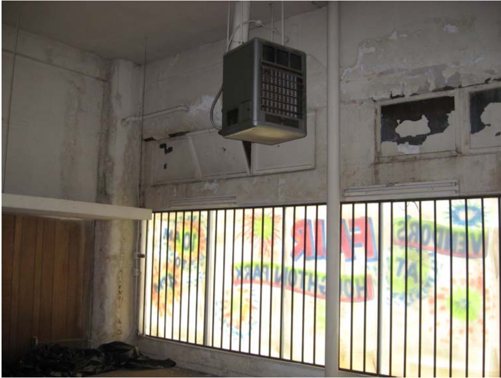
17. Water damage in the former furniture store.
