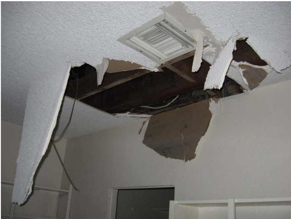
14. Water damage on the former church mezzanine level.
