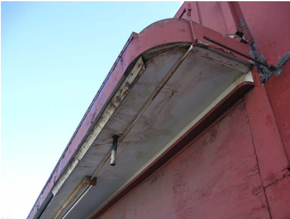
12. Poor condition of the overhand at the furniture store.
