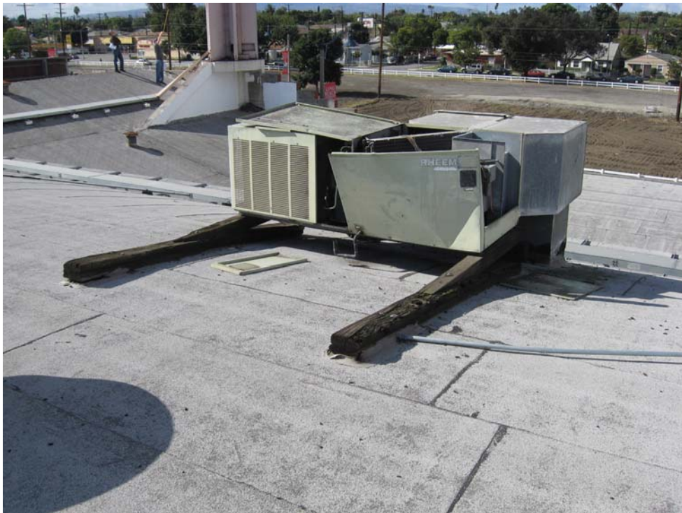
32. Vandalized mechanical equipment.
