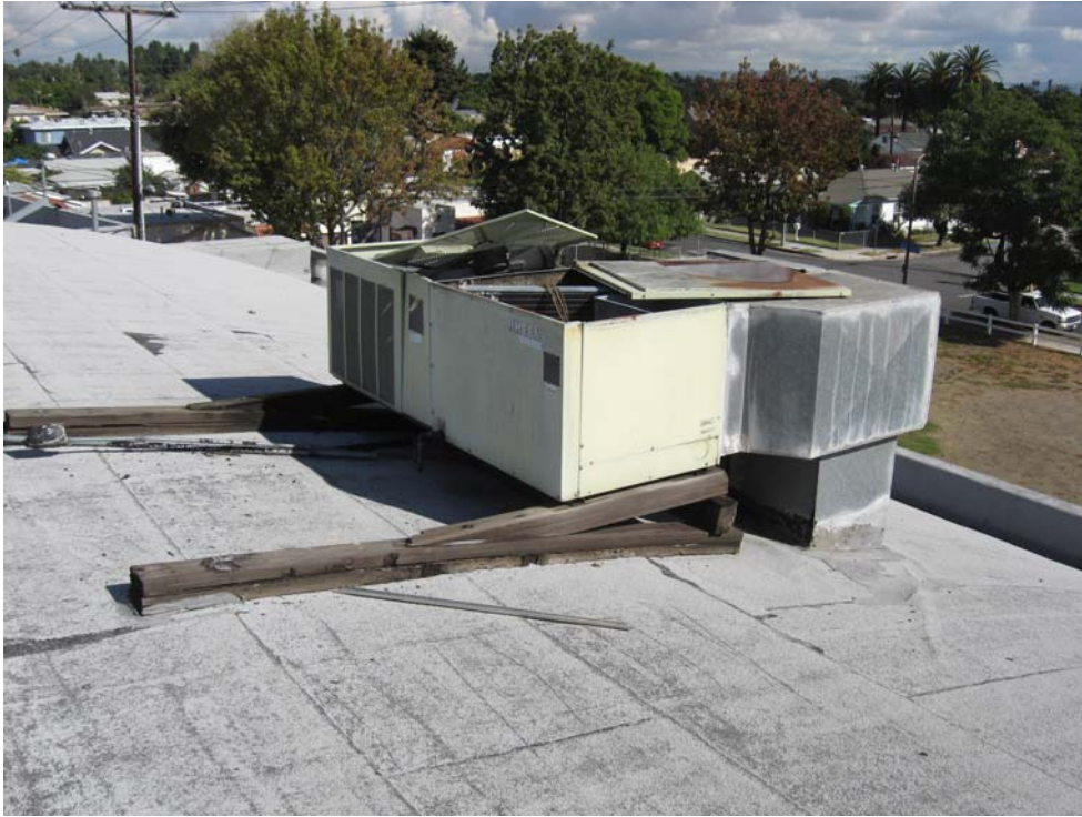
31. Mechanical units on the roof have been vandalized.
