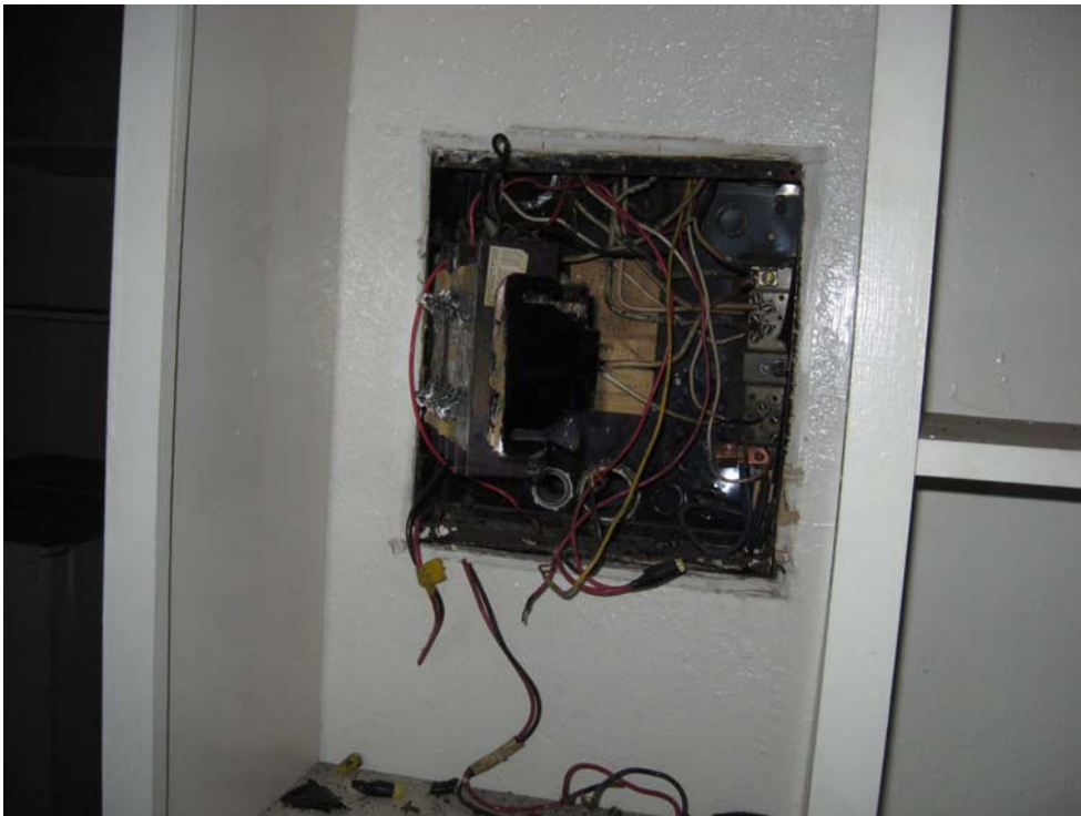
22. Electrical panel stripped of wires.
