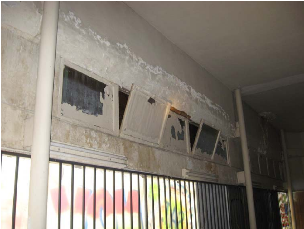
16. Water damage in the former furniture store.
