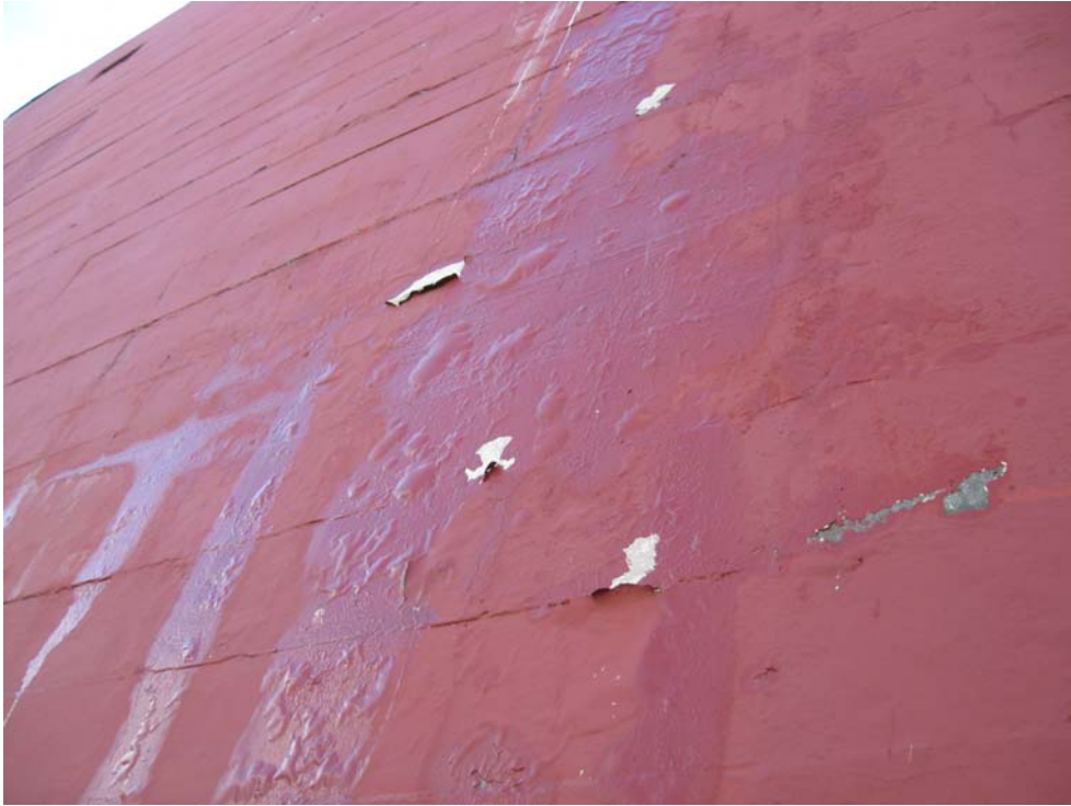
13. Water damage over the exterior wall.
