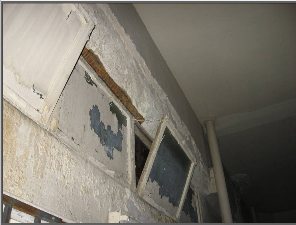
Photo 7: Water damage at interior face of west Hanson Building storefront.
