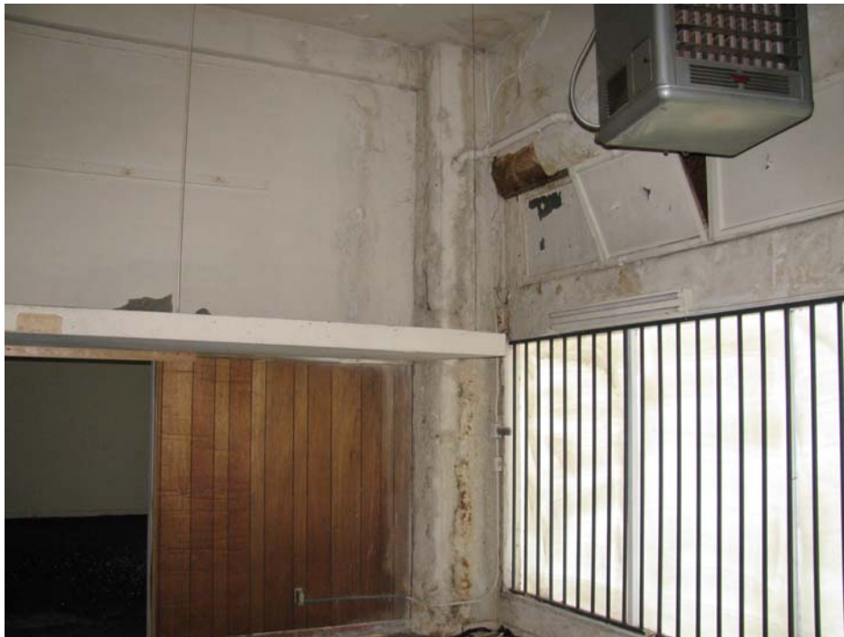
10. Water damage at the interior of the Hanson Building.
