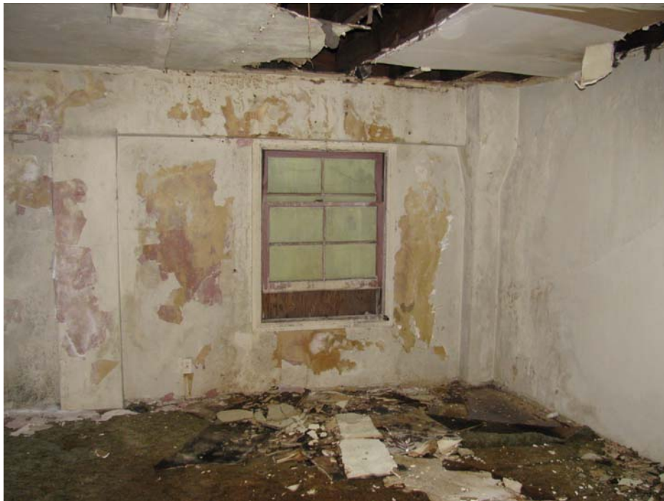
12. Water damage to wall and ceiling Hanson Building.
