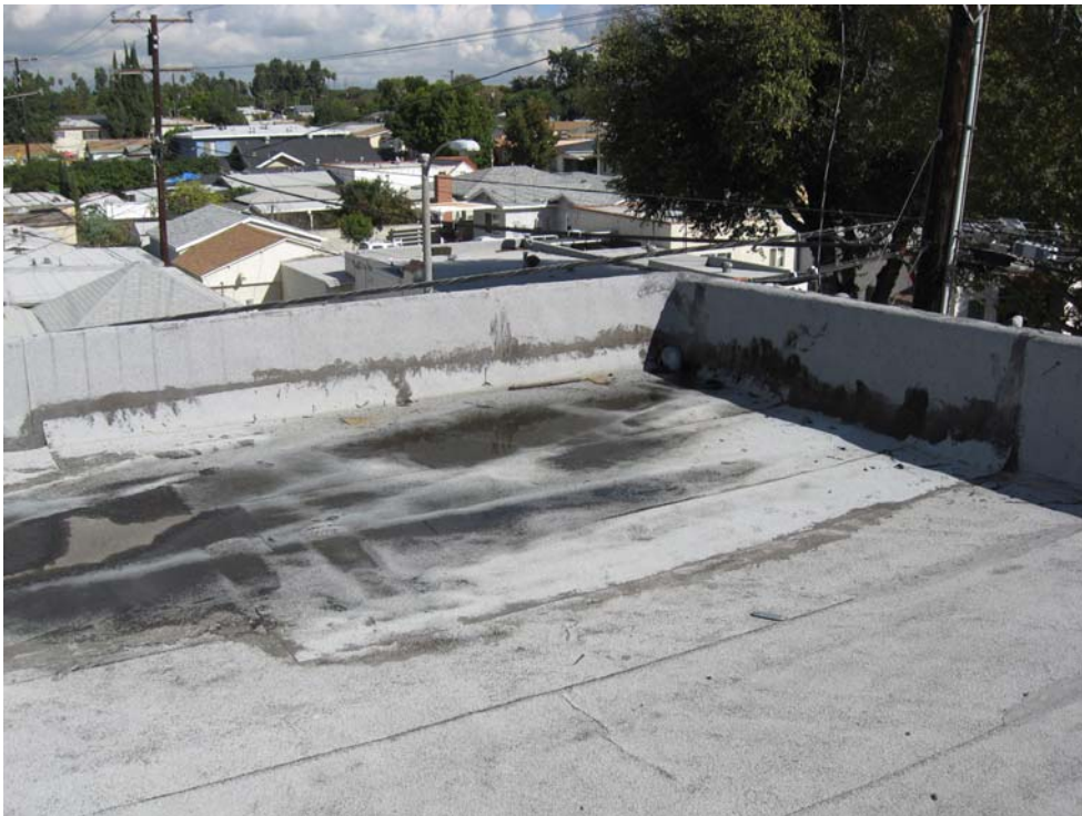
30. Poor condition of the roof.
