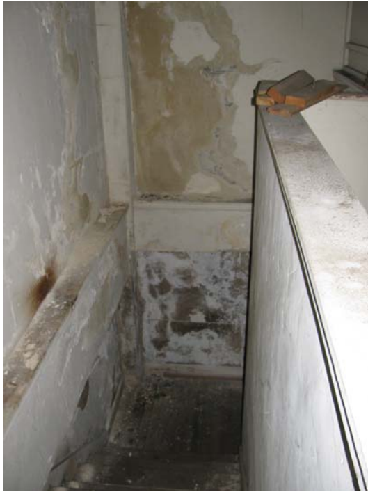
13. Water damage at stairway Hanson Building, not mold on walls.
