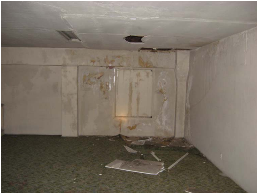
20. Active roof leak and damage inside former furniture store.
