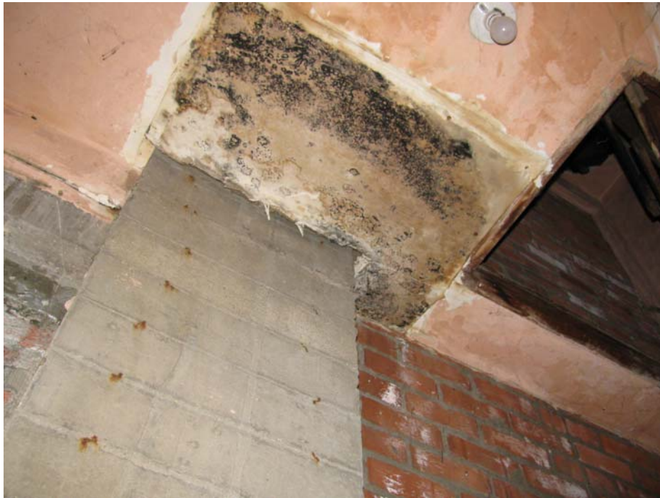
14. Mold at theater ceiling finishes.
