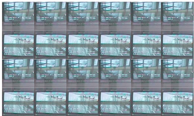
Fig. 3-29. Operation control center monitors
