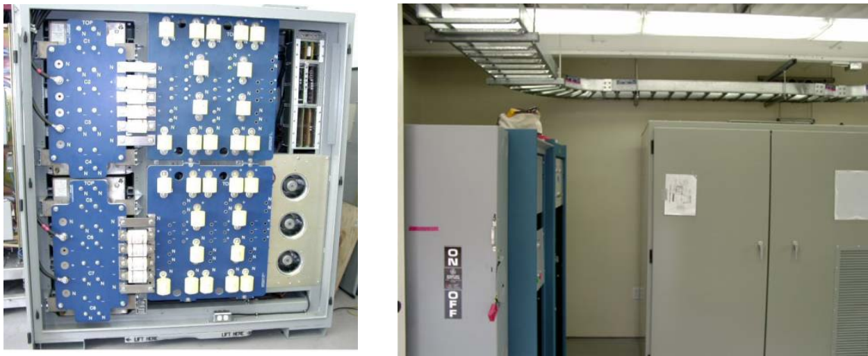
Fig. 3-22. Insulated gated bipolar transistor (IGBT)-based inverter module and urban maglev test track electrical room
