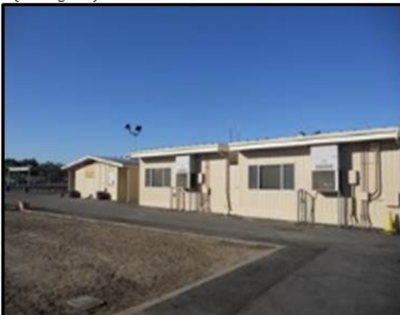
PHOTO 5: Dirt lot where centrally located building was removed/Portable buildings in background (looking southwest)
