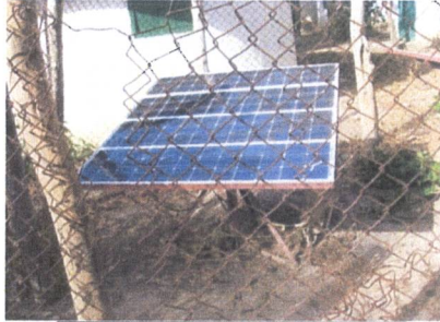
Solar Panel for pump
