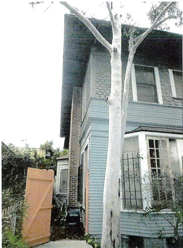
West elevation. 1938 bay window in front. Original bay on west side of first story.
