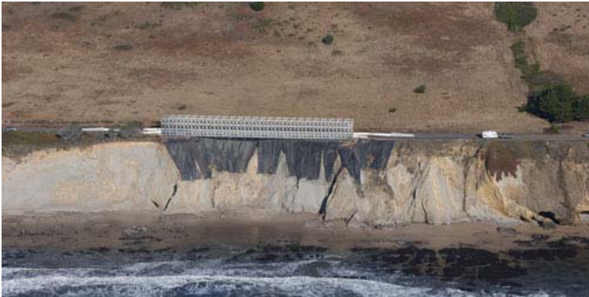
Figure 35. Road erosion along Highway 1 with deployment of erosion mitigation strategy
