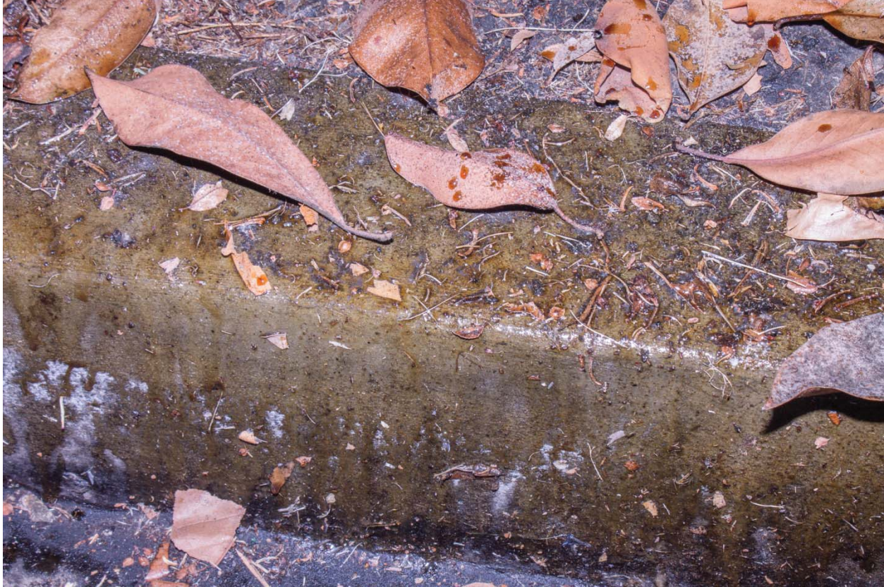
12. White surfaces like curbs appear as if they have been lacquered or varnished with shiny, amber-colored shellac.
