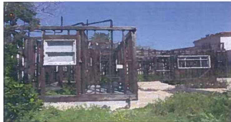
Figure 18: Rear elevation of 2810 E. 1 st Street, view to the north, March 9, 2011. Image courtesy of LSA Associates.
