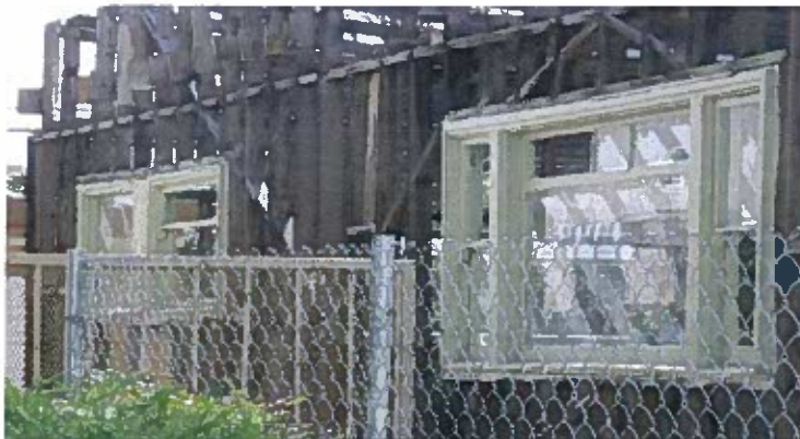
Figure 17: Window details at east side elevation, 2810 E. 1 st Street, view to the southwest, February 21, 2013. Source: GPA.
