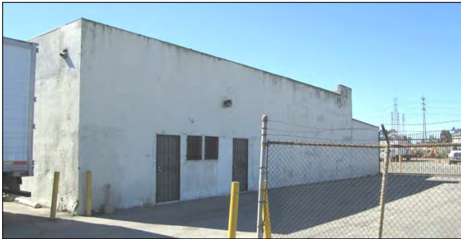
Detail of the north elevation of the western end of 6845 Atlantic Avenue, view to the southwest.
