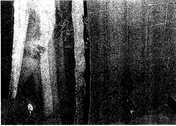
Mold, water damage
