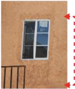
Caption: Changing window openings can leave "scars" on the exterior of a building. Red arrows indicate the original extent of the opening.
