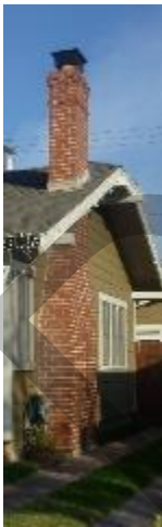
Caption: A chimney on a contributing property in the Bluff Heights Historic District.
