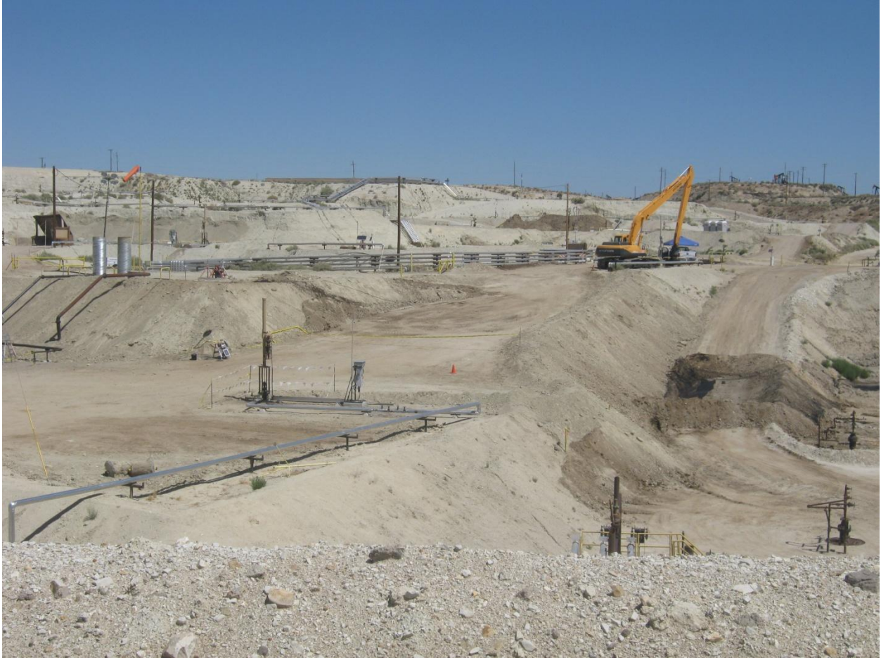
Photograph 14 – View of the June 27 reactivated surface expression location on TRC Operating Company’s “Bull” lease in relationship to the June 21 Chevron accident site and surface equipment of the subsurface containment structure. The reactivated surface expression is the bermed and netted area on the right. The accident site is 15 feet to 20 feet to the right of the wind sock pole. The surface equipment is on the left at the base of the slope. The two pipes running up the slope carry steam from the buried surface containment structure to be vented in the two silver cylinders. The boundary between Chevron and TRC is essentially the slope leading to the yellow excavator.
