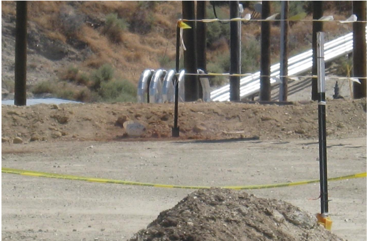
Photograph No. 11 - View of the accident spot. The victim's hard hat can be seen at the base of the berm at the edge of the sink hole.
