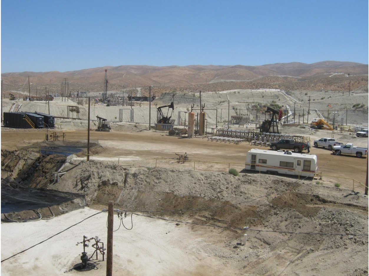
Photograph No. 13 – View of the TRC June 22 surface expression location in relationship to the June 21 Chevron accident site. The TRC surface expression is on the left and the accident site is on the right, approximately 40 yards beyond the yellow excavator, near the base of the orange wind sock’s pole. This surface expression was recorded as tilt meter event on June 22.
