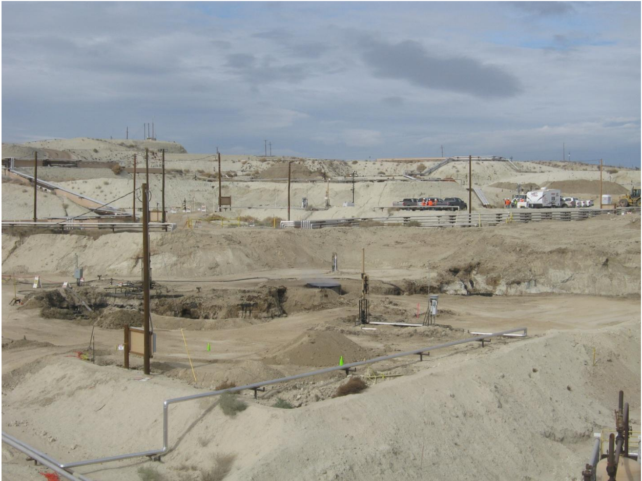
Photograph 28 – View of Well 20 surface expression area on January 20, 2012 after crater and terrace excavation. As seen in the middle of the photograph, a large diameter metal culvert has been placed over the crater vent. Trenches excavated to remove the radial drains can be seen extending from the culvert. Minor amounts of energy, in the form of bubbles, rise to the surface inside the trenches. The subsurface containment structure has not been excavated.
