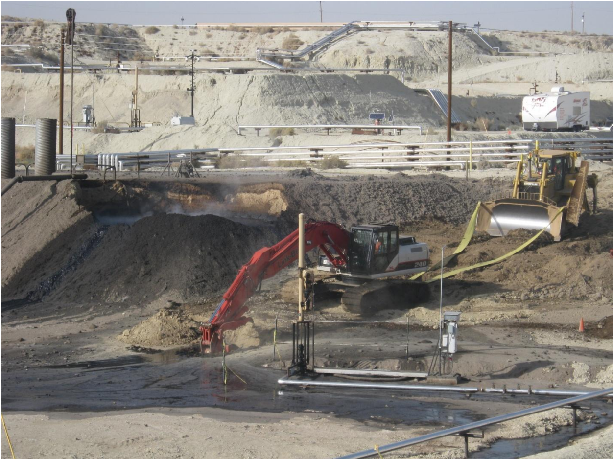
Photograph 27 – View of the start of investigative and remedial excavation of the Well 20 surface expression area on December 1, 2011. Spot locations were excavated to determine the stability of the ground and subsurface. No ground or subsurface instability was discovered.
