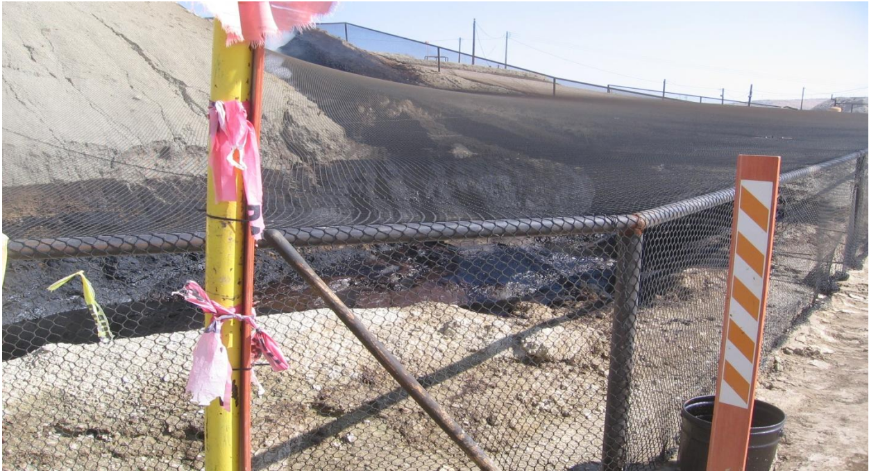
Photograph 2 - View of Chevron Well 20 surface expression site and fluid pit on 10/11/10. Location was continually active with surfacing water, oil and steam. A road at the end of the netting leads to the upper terrace.
