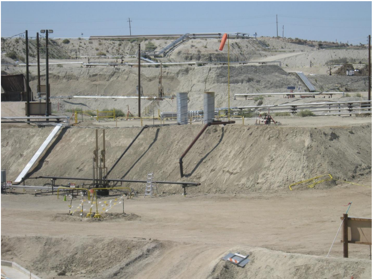
Photograph No. 9 - View of the surface equipment above the subsurface containment structure and remediated surface expression site on the day of the accident, June 21, 2011. The previous surface expression fluid pit was located at the base of the slope above where the present subsurface containment structure exists (the ladder in the picture is a good reference). The crater would have been somewhere between the right of the brown pipe running up the slope of the terrace and the corner of the upper terrace. Well K210 can be seen to the right of the yellow wind sock pole. The accident location is to the right of the wind sock pole approximately 15 feet to 20 feet, at the edge of the terrace. The two vertical cylinders on the upper terrace provide elevated steam release from the subsurface containment structure on the lower terrace. The road connecting the lower and upper terraces is at the extreme right of the picture.
