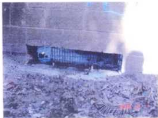
HOLE ALONG BLOCK WALL BETWEEN THE NURSERY AND PRIVATE PROPERTIES
