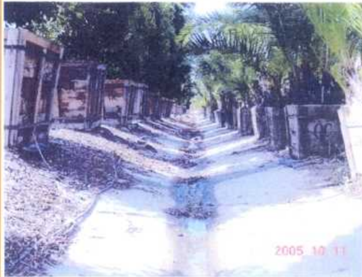
V-DITCH ON NURSERY SITE BEHIND BLOCK WALL
