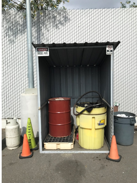
Photograph 5: Hazardous Materials Storage Area
