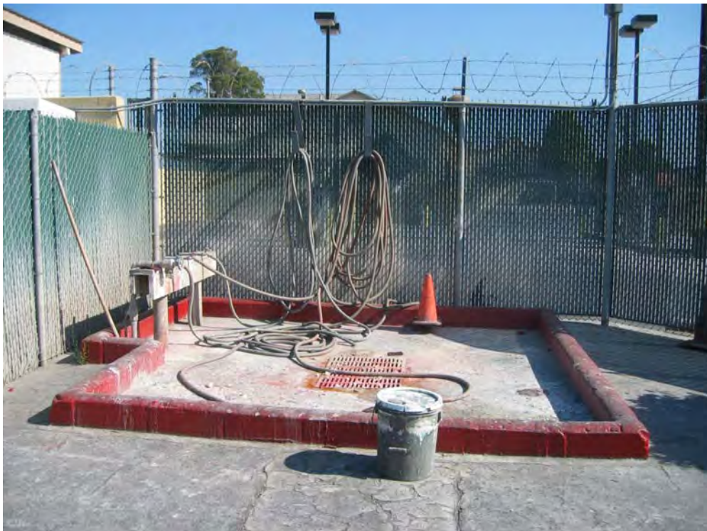
Photo 16. Clarifier for Paint Equipment Rinse Water on APN 7271-008-901.
