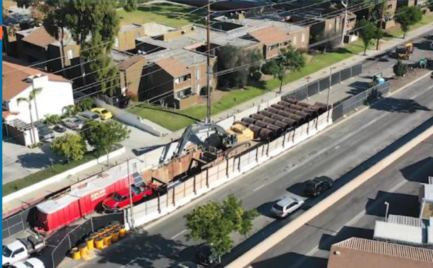
Second Lower Feeder Access Site Photo courtesy of Black & Veatch, 78" steel water pipe
