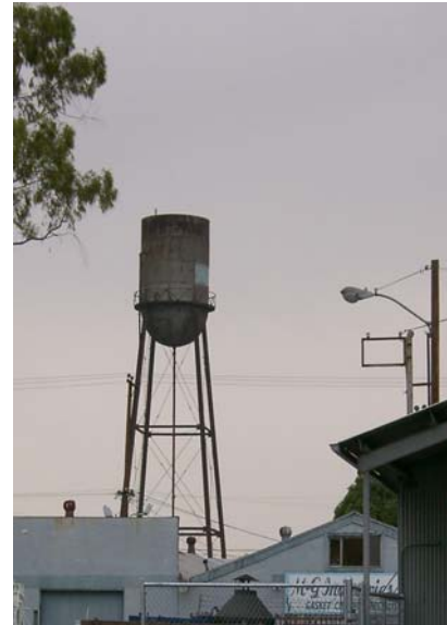
Restoring the SnugTop water tower is an important step in creating a highly visible icon for Westside.
