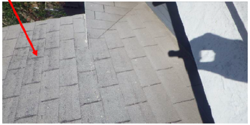
*Wear/granulation deterioration at the roof shingles
