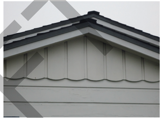
Scalloped edges in gable ends
