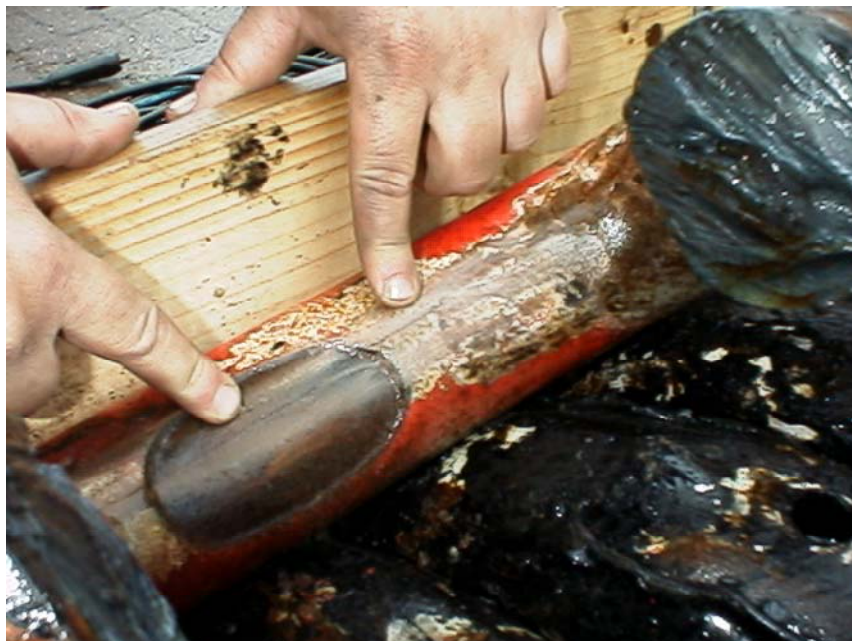
Figure 7-3 Crack initiated in the stud foot print (DNV photo).
