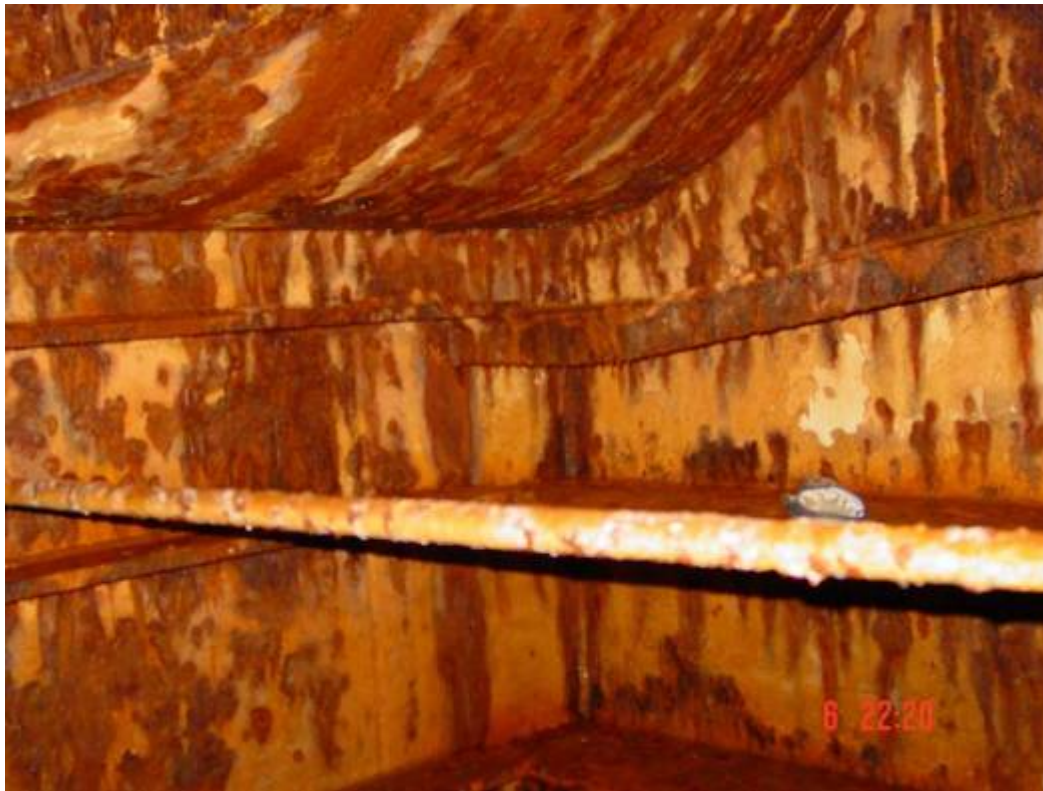
Figure 3-2-3 General Corrosion inside ballast tank (DNV photo).
