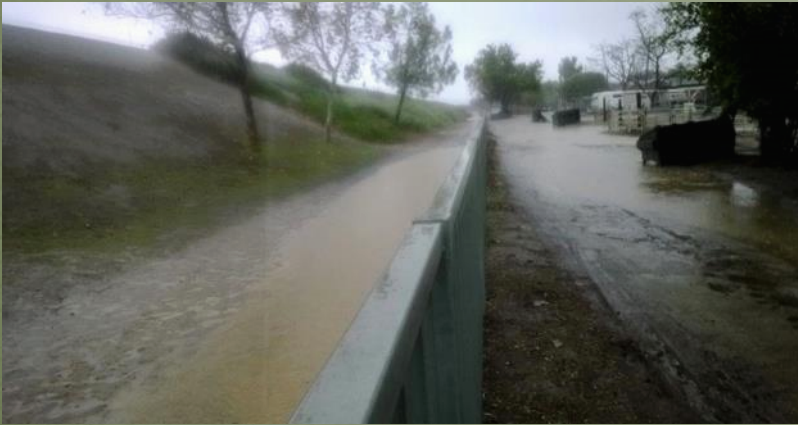
Run-off at Toe of Levee
