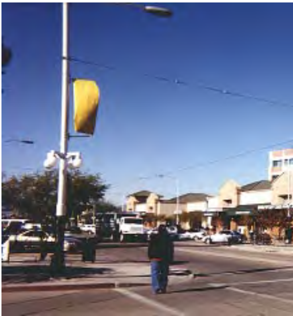
Example of pedestrian-oriented lighting mounted on hi-mast poles, University Boulevard, Tucson, Arizona.
